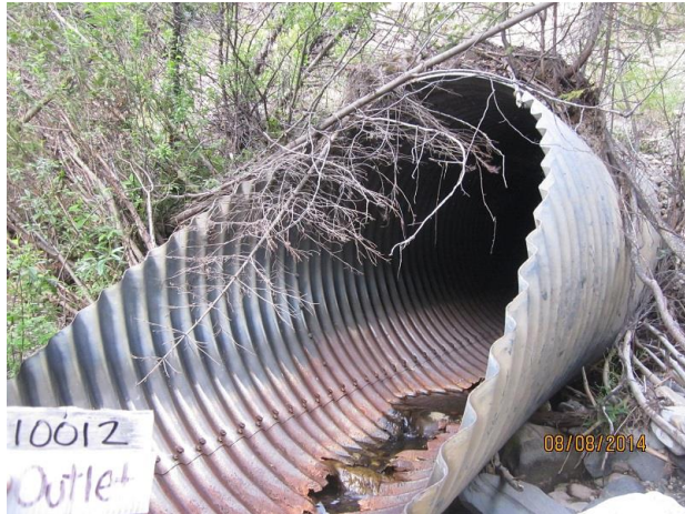
Photo 19, Site 10012 – Outlet perched 0.3m and rusted.
