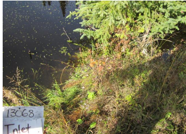
Photo 10, Site 13068 – Culvert inlet obstructed with large beaver pond upstream.
