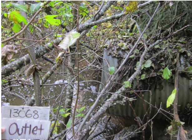
Photo 9, Site 13068 – Outlet drop of 0.4m.
