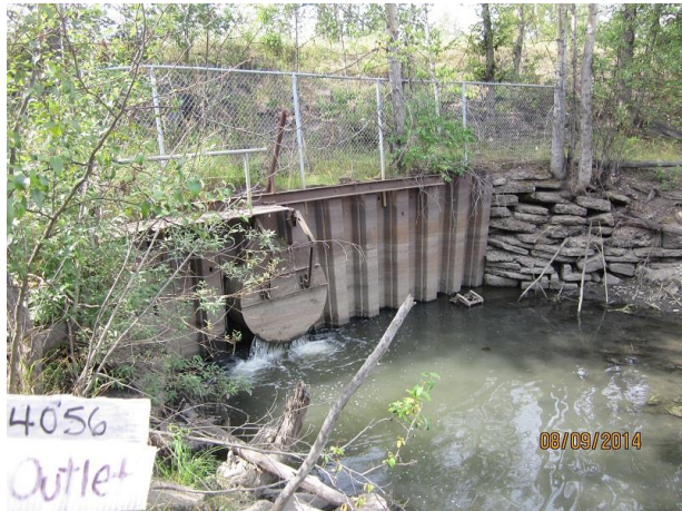
Photo 15, Site 4056 – 0.3m perched culvert with outlet backflow control structure (for Fraser River).
