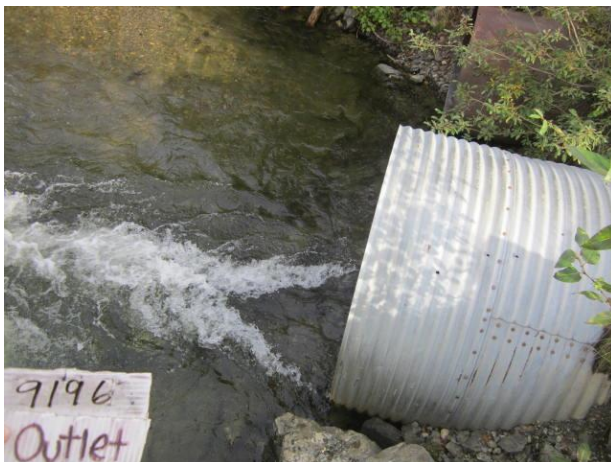
Photo 5, Site 9196 – High value habitat, perched culvert 0.5m
