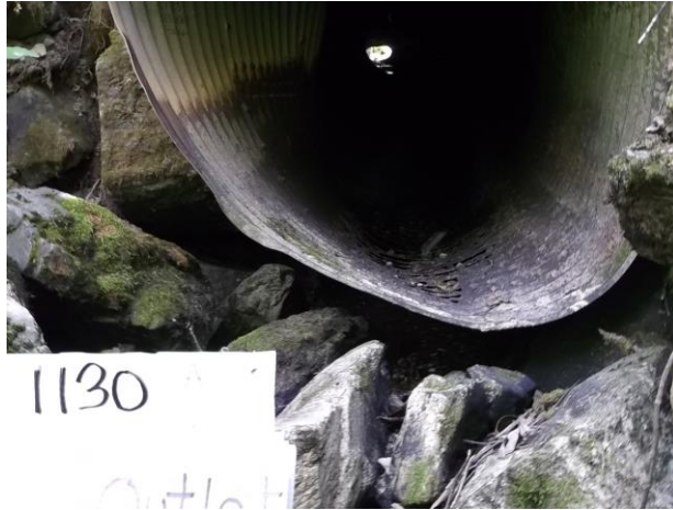
Photo 13, Site 1130 – Culvert outlet perched and rusted through resulting in no flow at the end of
