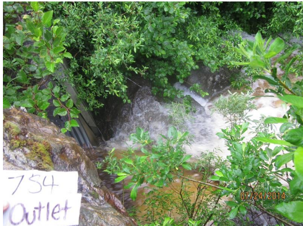
Photo 21, Site 784 – Culvert outlet perched 1.0m,
