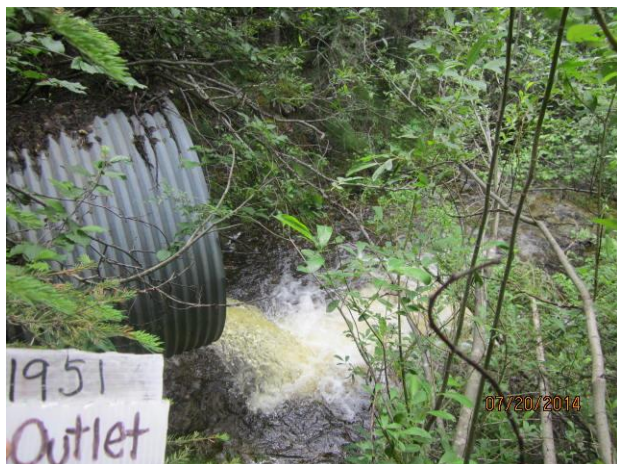
Photo 23, Site 1951 – Culvert outlet perched 1.1m.
