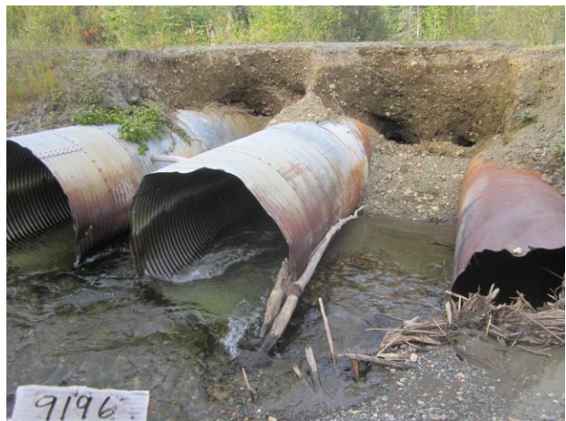
Photo 6, Site 9196 – Culvert inlets partially washed out.
