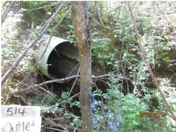
Photo 11, Site 514 - Culvert outlet drop of 0.34m
