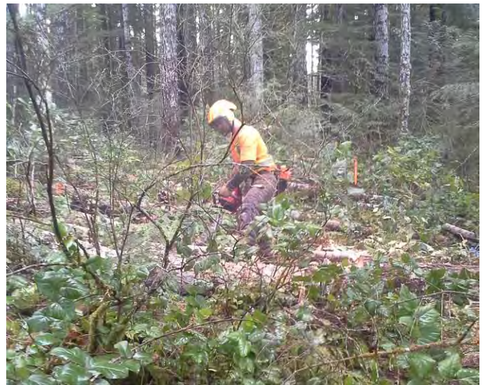
Photo 4. Falling hazard trees, trail right-of-way and South Tower location. February 23, 2016.
