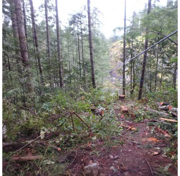
Photo 14. Looking out along the newly installed skyline towards the north cliff face, March 23, 2016.
