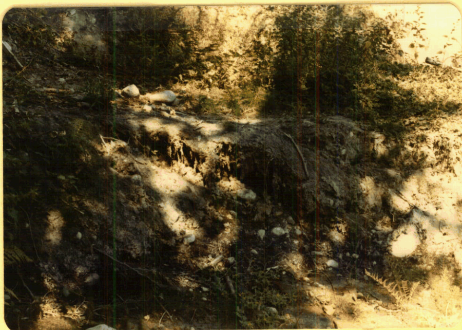
Looking southeast behind slump area.
