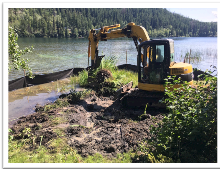
Figure 2. Photo of the silt fence and excavator removing Yellow Flag Iris on Tyaughton Lake.
