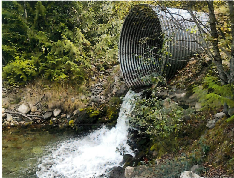
Figure # 1 - Culvert under Highway 6 – September 2014
