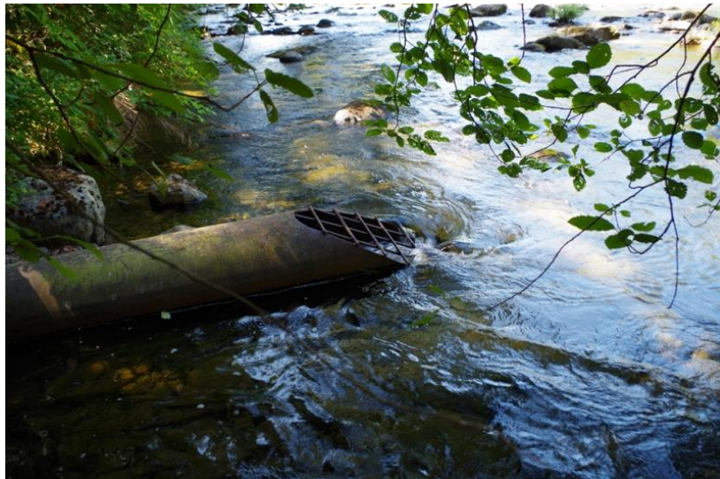
Photo 1. Forbidden side-channel intake at Puntledge River, upstream of HWY 19.
