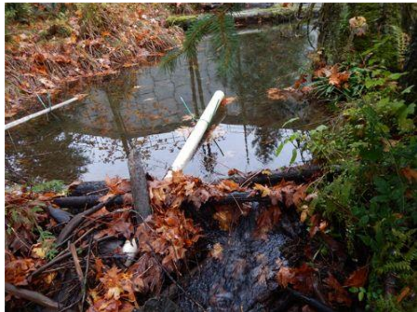
Photo 2. Beaver pipes installed at the upstream end of Forbidden side-channel to maintain flow.
