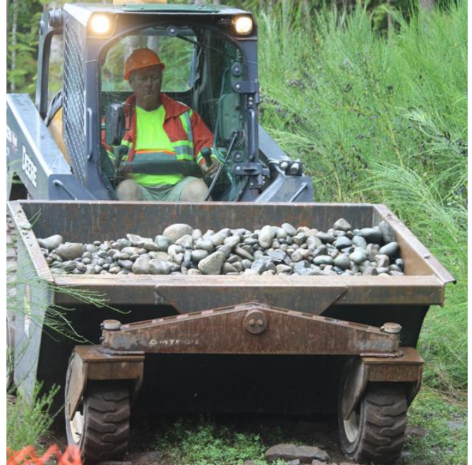
Photo 6. Tracked Skidsteer with wheelbarrow attachment to move gravel to trolley loading location.
