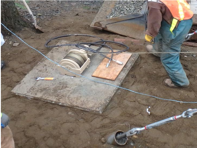
Photo 1. Installed hydraulic winch used to deploy and retrieve gravel trolley.
