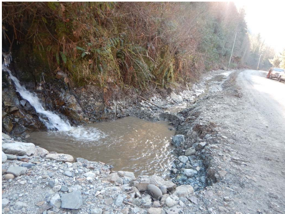
Realignment of roadside ditch/channel on east side of Forest Service Road (facing south; water flowing south into Branch 100 Creek culvert)
