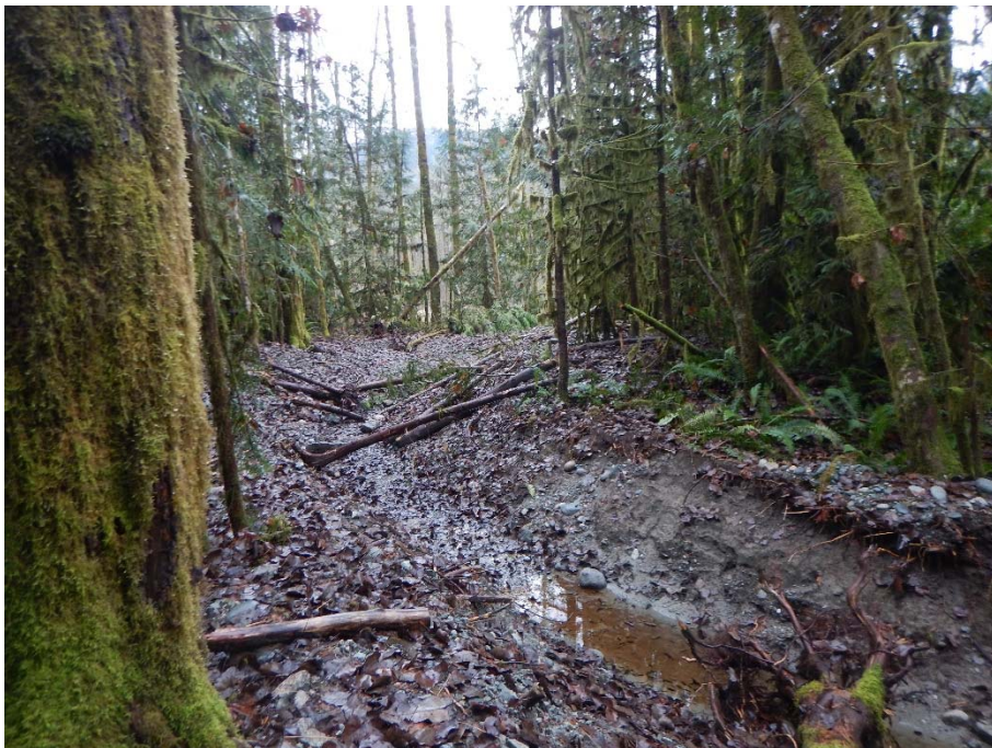
Facing west towards newly constructed channel that will connect with Mile 22 Creek culvert
