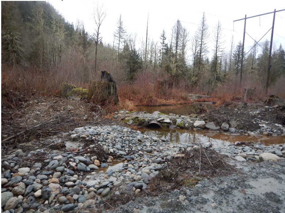
Facing north, new channel construction and culvert installation along north side of road
