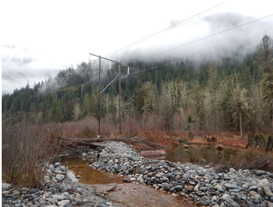
Facing north just above "Culvert 2" at new culvert to improve flows and prevent beaver obstructions
