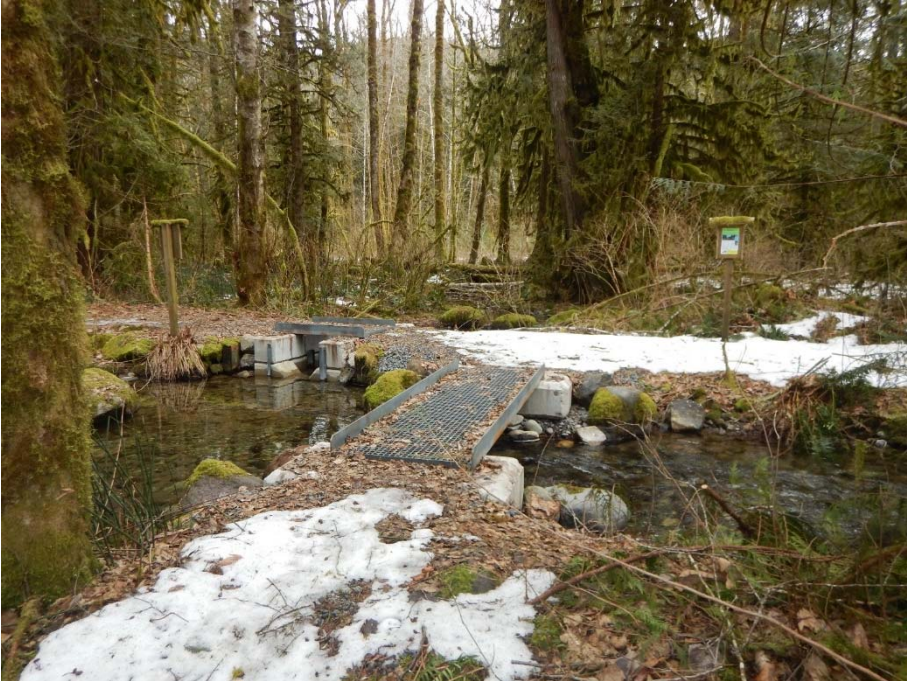
Birth of a Stream South – replaced foot bridges, replaced weir, in-stream flow diversion structures
