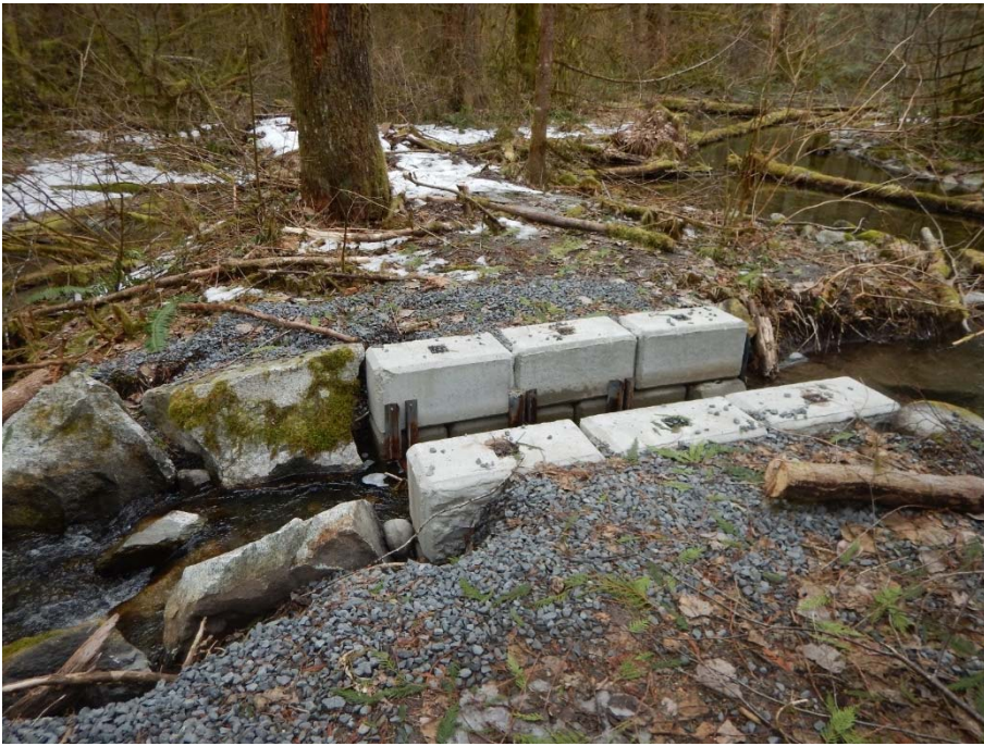
Coho Connector – replaced weir with lock blocks and new in-stream flow structure
