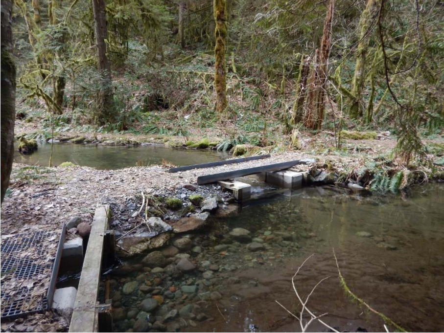
Birth of a Stream South – replaced foot bridges and weir and improvements to flow structures
