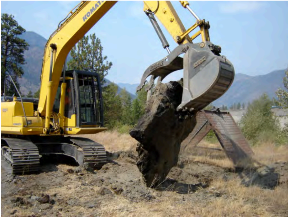
Figure 5 Asphalt chunk being dug up - evidence of MOT operations - this area continues to be difficult to plant into August 2009
