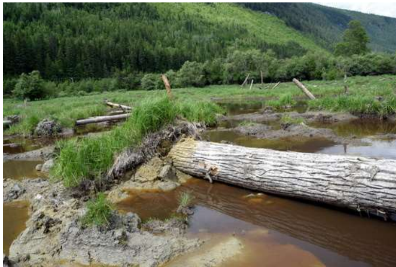
Large diameter logs would be placed in the restored wetlands to resemble trees naturally falling over. This photo shows one of many dead trees placed in wetlands restored at Meadow Creek in January 2016.
