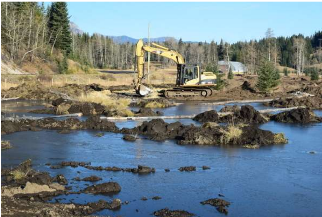
This photo shows an emergent wetland under construction near Fernie, British Columbia. Note the ridges and logs being placed in the basin.
