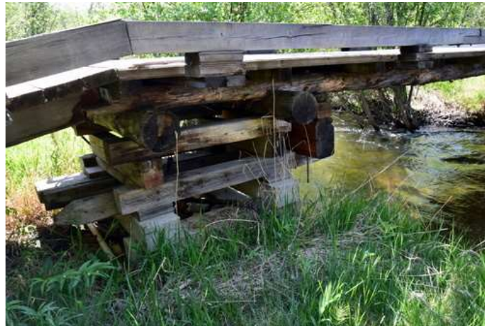
The bridge was not designed for heavy equipment to cross
