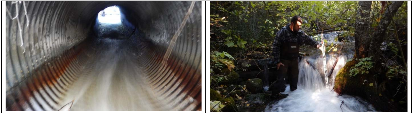
Figure 14. Left: Depth and velocity conditions inside the BCH RoW crossing of Blackwater Creek were characterized by sheet flow conditions, which did not meet criteria for fish passage. Right: Drop heights, and pool depth to jump height ratios associated with weirs downstream of the BCH RoW crossing of Blackwater Creek did not meet criteria for fish passage.
