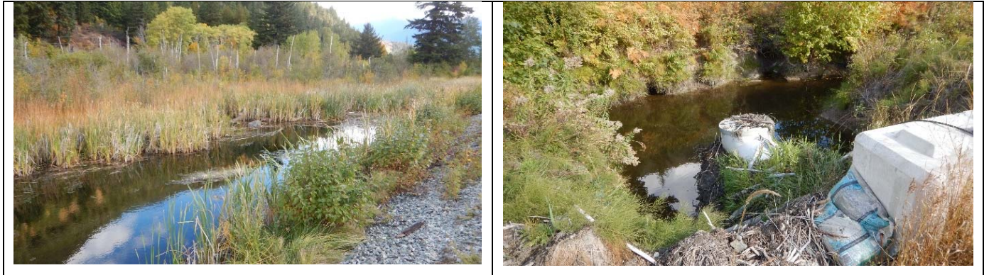
Figure 9. Left: open water wetland upstream (north) of the CN Track on 9484 Portage Road, and west of the BPAO. A second wetland is also located on the south side of the track in this area. Right: Beaver proof add-on (BPAO) attached to the upstream end of the CN culvert. Despite the name this structure is still affected by beaver activity. s
