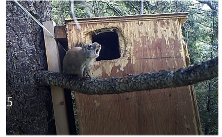
Photograph A: example of squirrel chewing damage.
