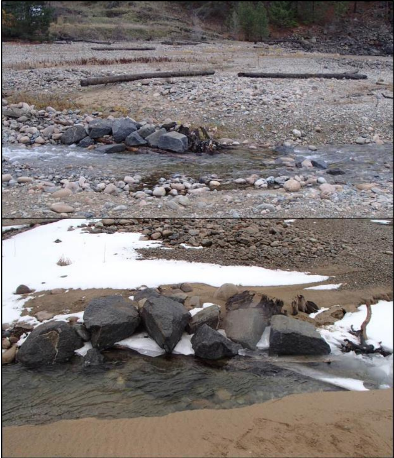
Figure 27. (Top) Structure 8 post -construction in November 2015; (bottom) Structure 8 in March 2018 after two years of being subjected to freshet and reservoir inundation. Photos by Evan Smith, Okanagan Nation Alliance, November 2015 and March 2018).
