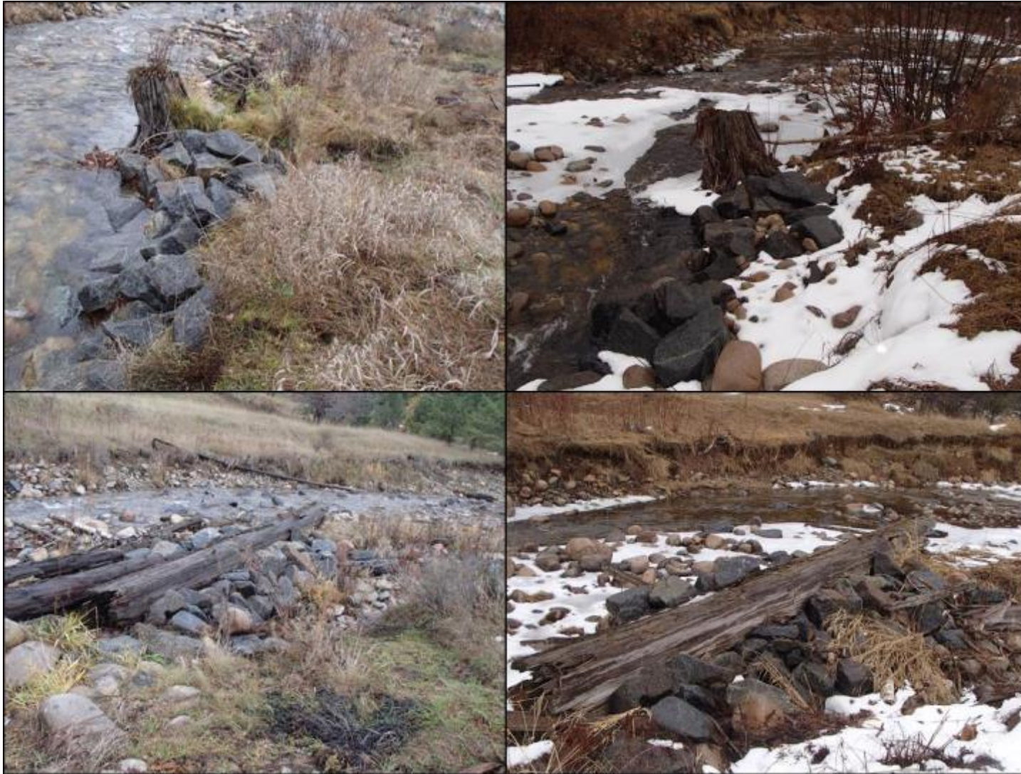
Figure 21. (Top Left) Structure 1 post -construction in November 2015; (top right) Structure 1 in March 2018 after two years of being subjected to freshet and reservoir inundation; (bottom left) Structure 2 post-construction in November 2015; (bottom right) Structure 2 in March 2018 after two years of being subjected to freshet and reservoir inundation. Photos by Evan Smith, Okanagan Nation Alliance, November 2015 and March 2018).
