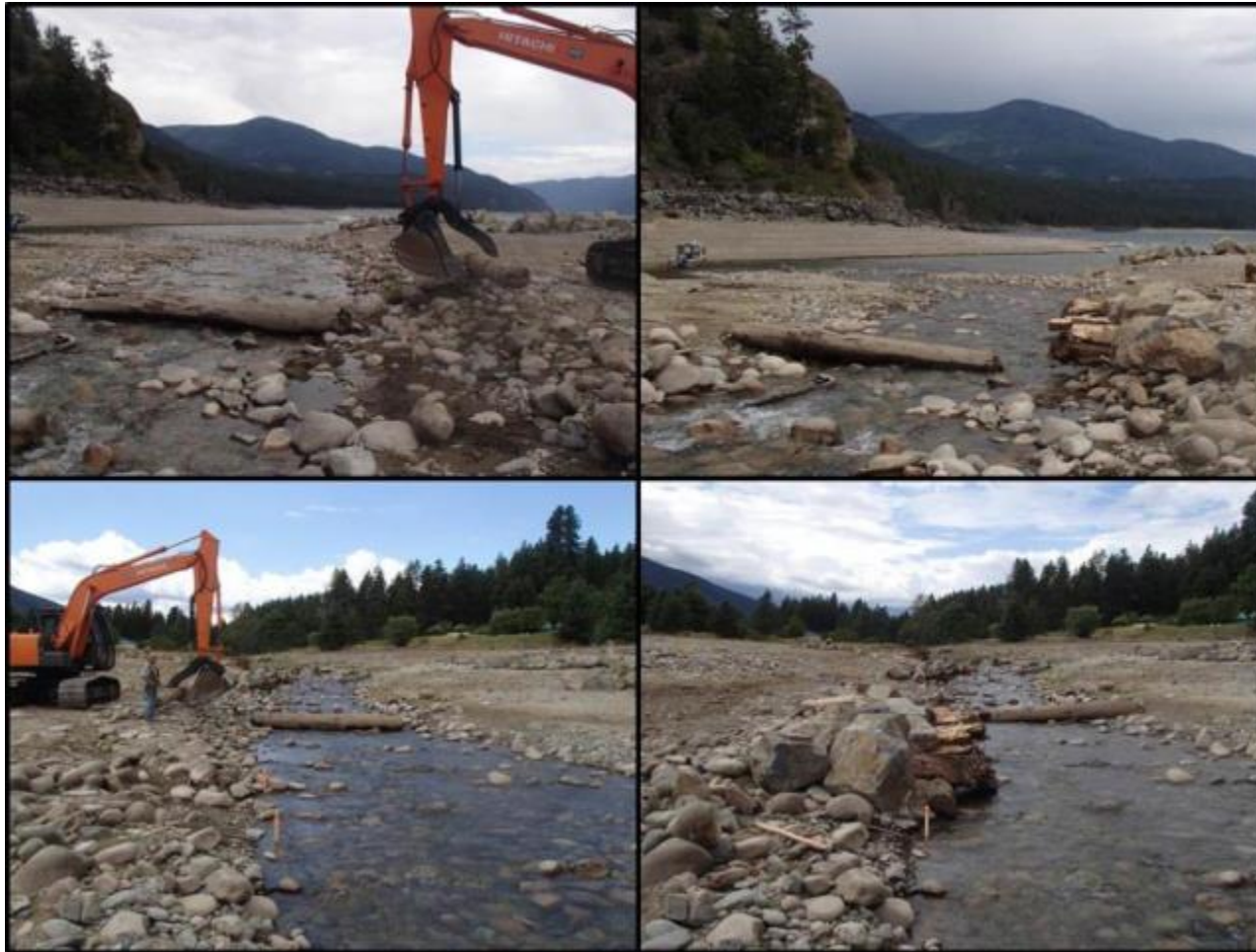
Figure 10. Before (top left and bottom left) and after (top right and bottom right) comparison from upstream and downstream perspectives, respectively, of Structure 12 on the right bank in the Deer Creek drawdown zone Photos by Evan Smith, Okanagan Nation Alliance, August 2016.
