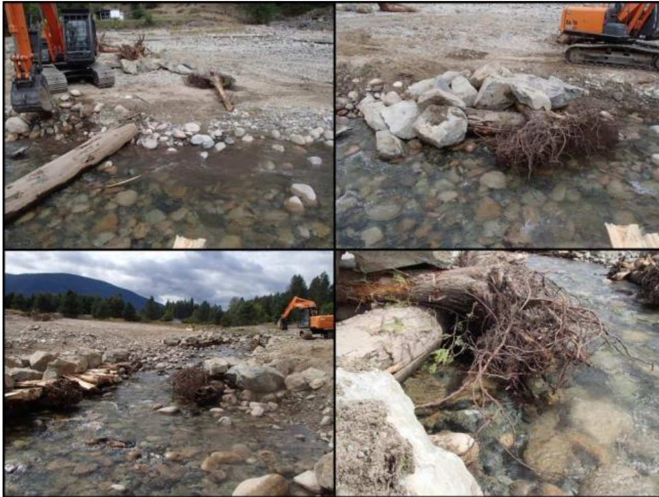
Figure 11. Before (top left) and after (top right) comparison of Structure 13 on the left bank in the section of Deer Creek within the drawdown zone from across the stream; (bottom left) a downstream perspective of Structure 13 in relation to Structure 12; (bottom right) a close up of Structure 13 from an upstream perspective depicting its effectiveness of creating pools and cover for fish. Photos by Evan Smith, Okanagan Nation Alliance, August 2016.
