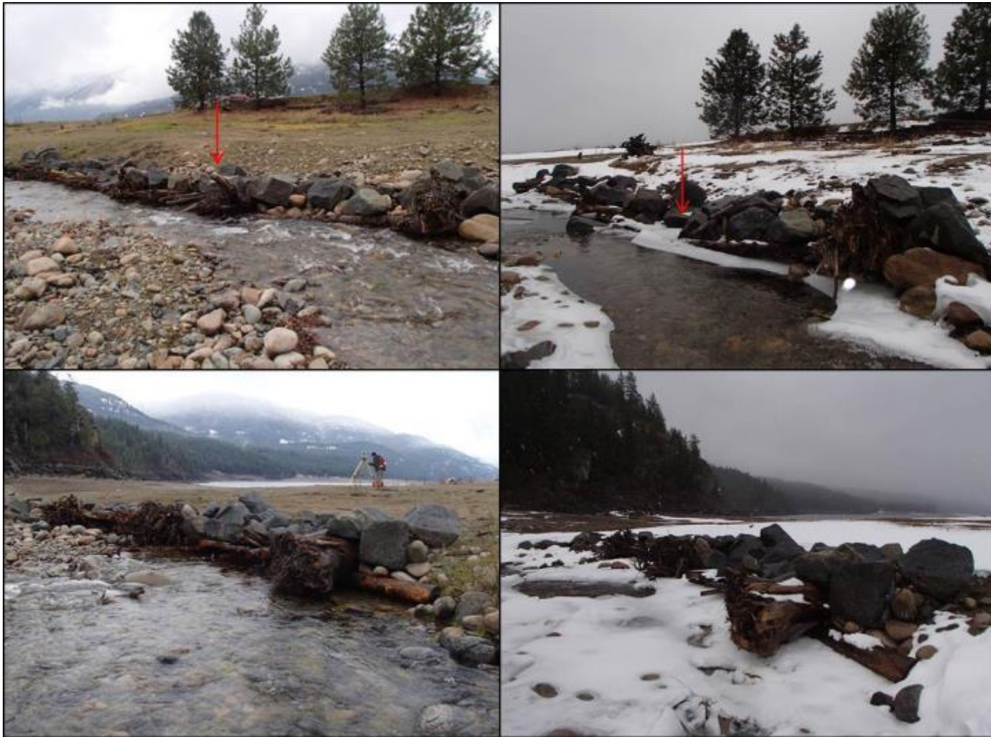
Figure 25. (Top Left) upstream portion of Structure 6 post -construction in November 2015 with red arrow highlighting Root 2; (top right) upstream portion of Structure 6 in March 2018 after two years of being subjected to freshet and reservoir inundation with red arrow highlighting the absence of Root 2; (bottom left) downstream portion of Structure 6 post-construction in November 2015; (bottom right) downstream portion of Structure 6 in March 2018 after two years of being subjected to freshet and reservoir inundation. Photos by Evan Smith, Okanagan Nation Alliance, November 2015 and March 2018).
