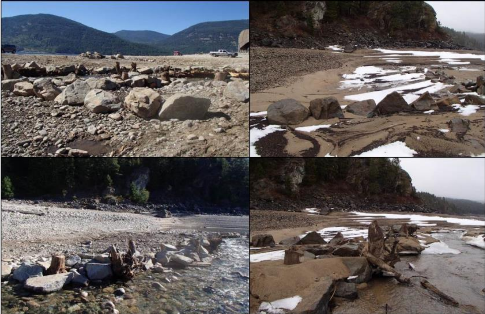
Figure 31. (Top Left) Structure 15 post -construction in August 2016; (top right) Structure 15 in March 2018 after one year of being subjected to freshet and reservoir inundation; (bottom left) Structure 16 post-construction in August 2016; (bottom right) Structure 16 in March 2018 after one year of being subjected to freshet and reservoir inundation. Photos by Evan Smith, Okanagan Nation Alliance, August 2016 and March 2018).
