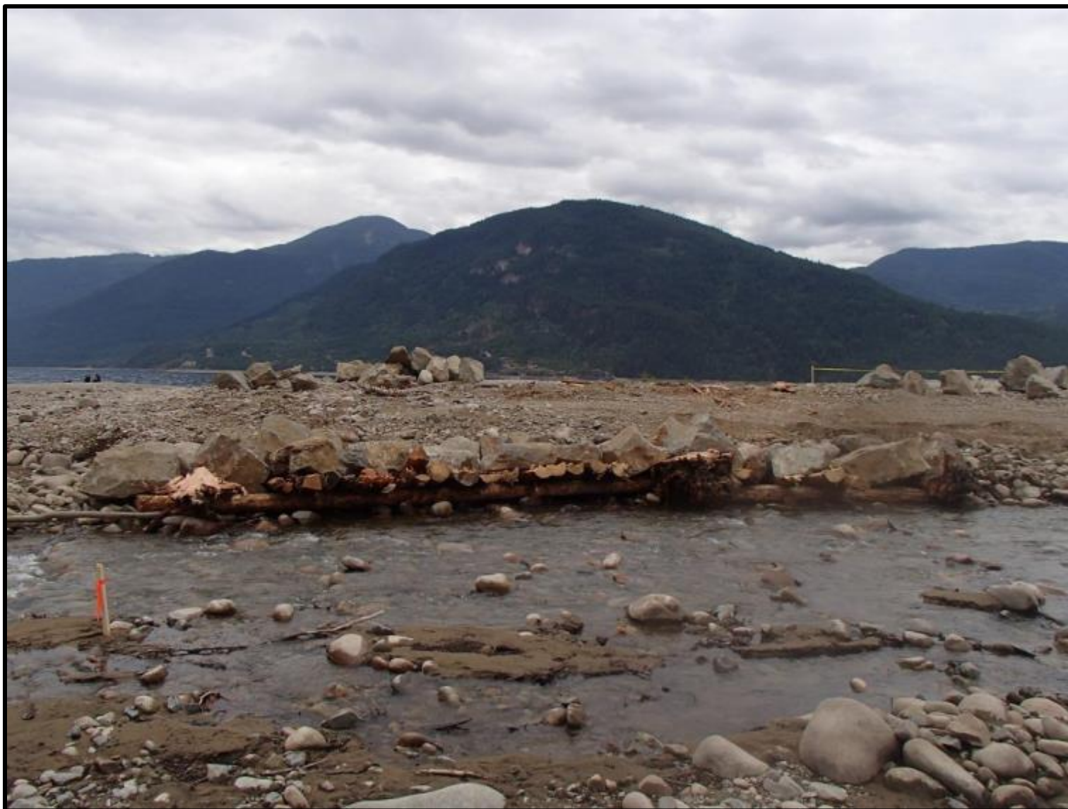
Figure 42. Structure 12 post-construction from across the stream on August 10 th 2016 . Photo by Evan Smith, August 2016.
