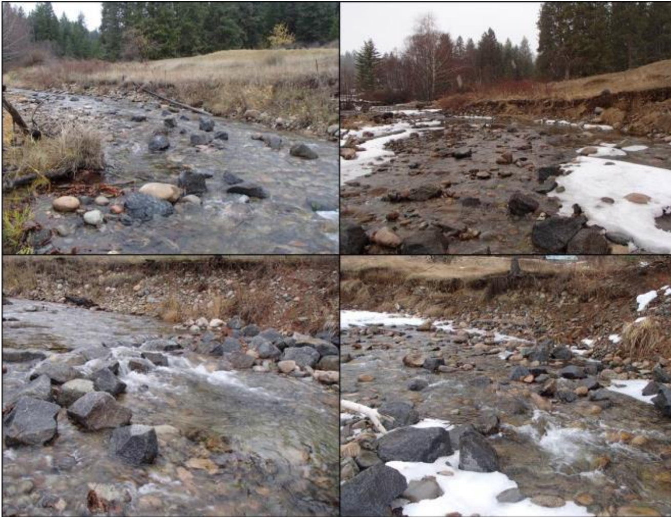
Figure 22. (Top Left) Structure 3 post -construction in November 2015; (top right) Structure 3 in March 2018 after two years of being subjected to freshet and reservoir inundation; (bottom left) Structure 4 post-construction in November 2015; (bottom right) Structure 4 in March 2018 after two years of being subjected to freshet and reservoir inundation. Photos by Evan Smith, Okanagan Nation Alliance, November 2015 and March 2018).
