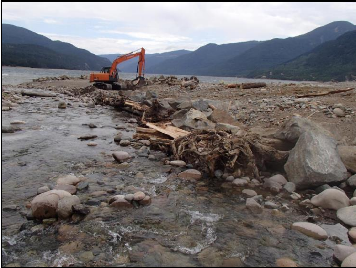
Figure 39. Structure 9 post-construction from an upstream perspective on August 9 th 2016. Photo by Evan Smith, Okanagan Nation Alliance, August 2016.
