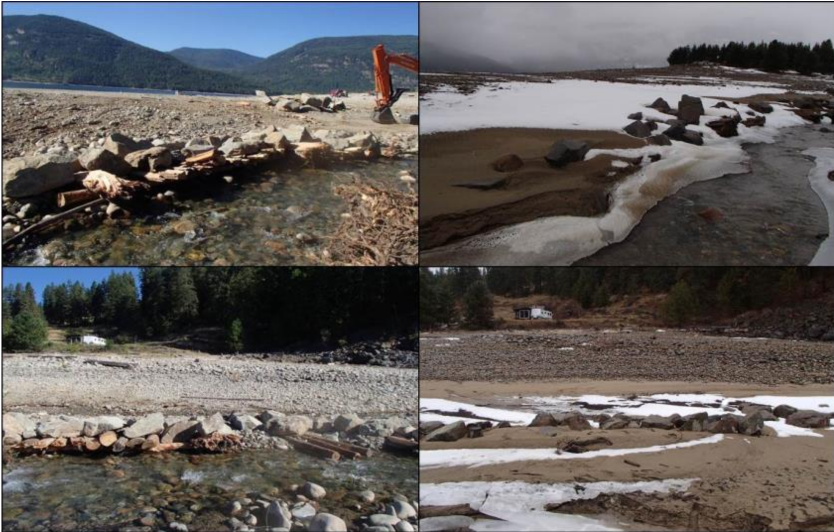
Figure 32. (Top Left) Structure 17 post -construction in August 2016; (top right) Structure 17 in March 2018 after one year of being subjected to freshet and reservoir inundation; (bottom left) Structure 18 post-construction in August 2016; (bottom right) Structure 18 in March 2018 after one year of being subjected to freshet and reservoir inundation. Photos by Evan Smith, Okanagan Nation Alliance, August 2016 and March 2018).
