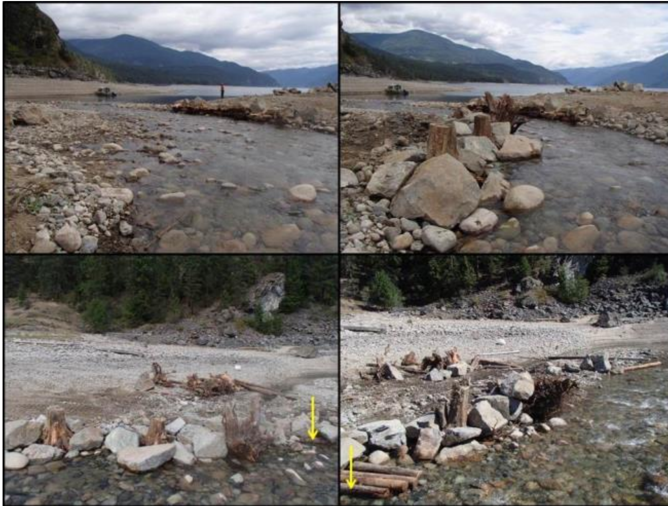
Figure 13. Before (top left) and after (top right) comparison of Structure 16 from an upstream perspective located on the left bank of the Deer Creek drawdown zone; (bottom left) view of Structure 16 from across the stream; (bottom right) continuation of Structure 16 from across the stream (point of reference indicated via yellow arrows. Photos by Evan Smith, Okanagan Nation Alliance, August 2016.
