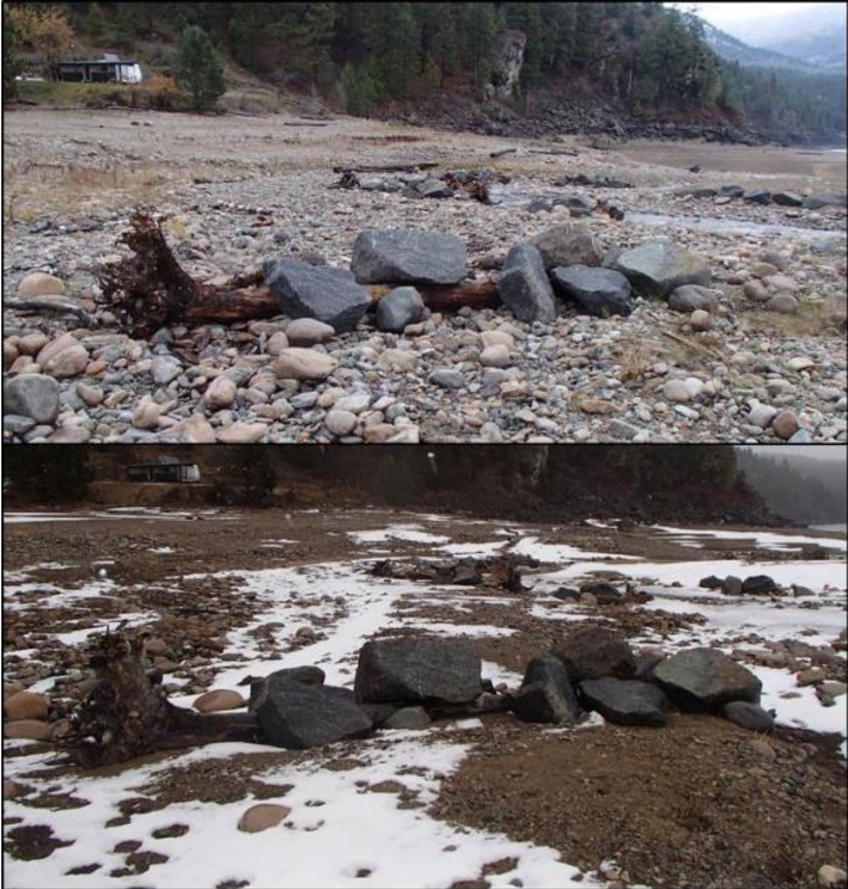
Figure 24. (Top) Structure 5a post -construction in November 2015; (bottom) Structure 5 in March 2018 after two years of being subjected to freshet and reservoir inundation. Photos by Evan Smith, Okanagan Nation Alliance, November 2015 and March 2018).
