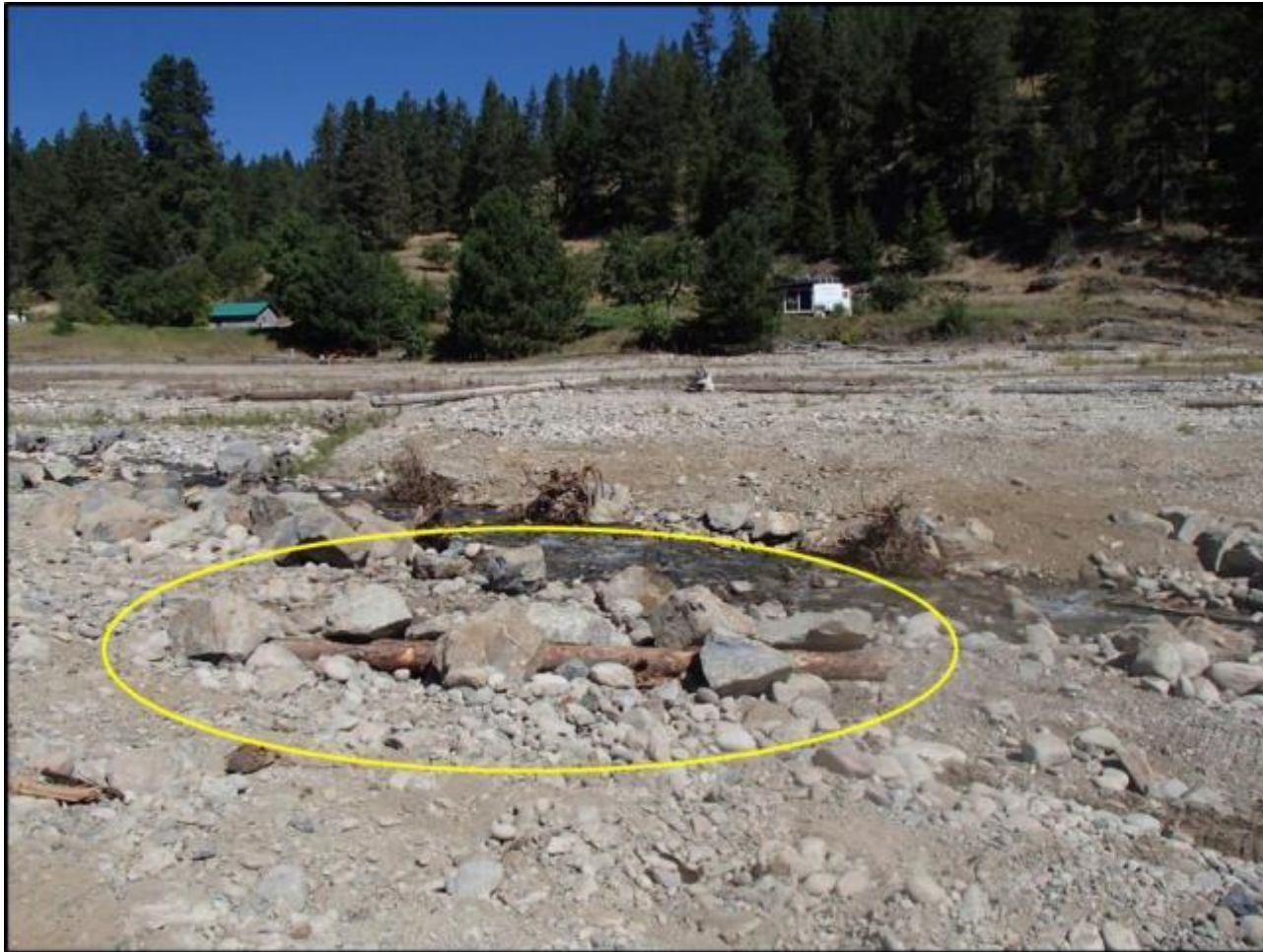
Figure 9. Structure 11 from a right bank perspective designed to deflect water into the original stream bed as higher flows recede. Photo by Evan Smith, Okanagan Nation Alliance, August 2016.
