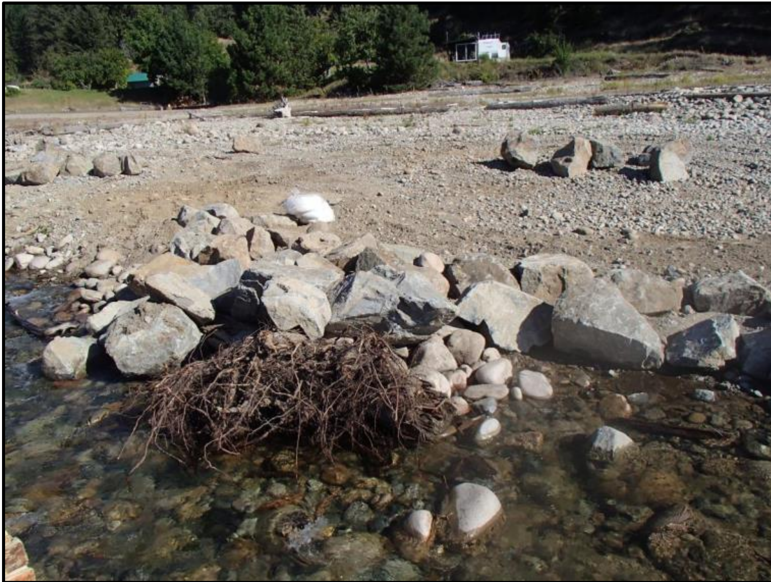
Figure 43. Structure 13 post-construction from across the stream on August 12 th 2016. Photo by Evan Smith, Okanagan Nation Alliance, August 2016.
