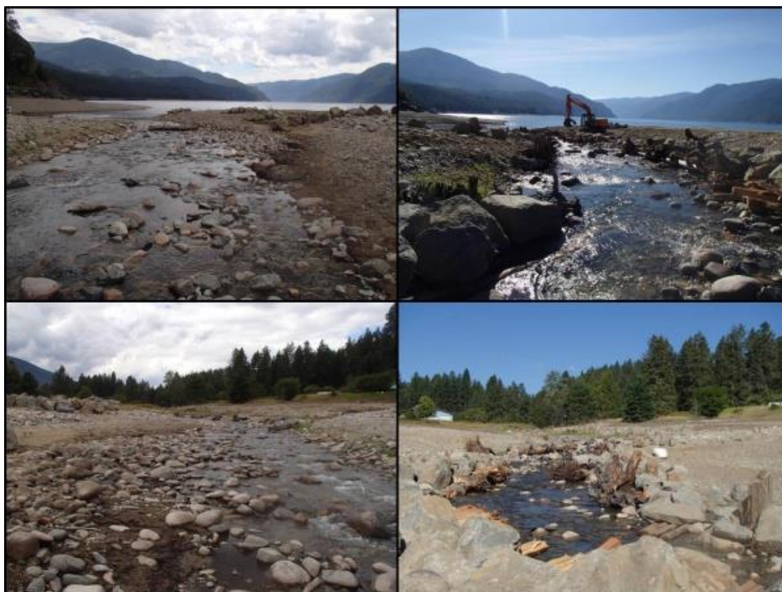
Figure 4. A downstream perspective from Phase I of Phase II before (top left) and after (top right) structure construction, and an upstream perspective from within the drawdown zone of Phase II before (bottom left) and after (bottom right) structure construction Photos by Evan Smith, Okanagan Nation Alliance, August 2016.
