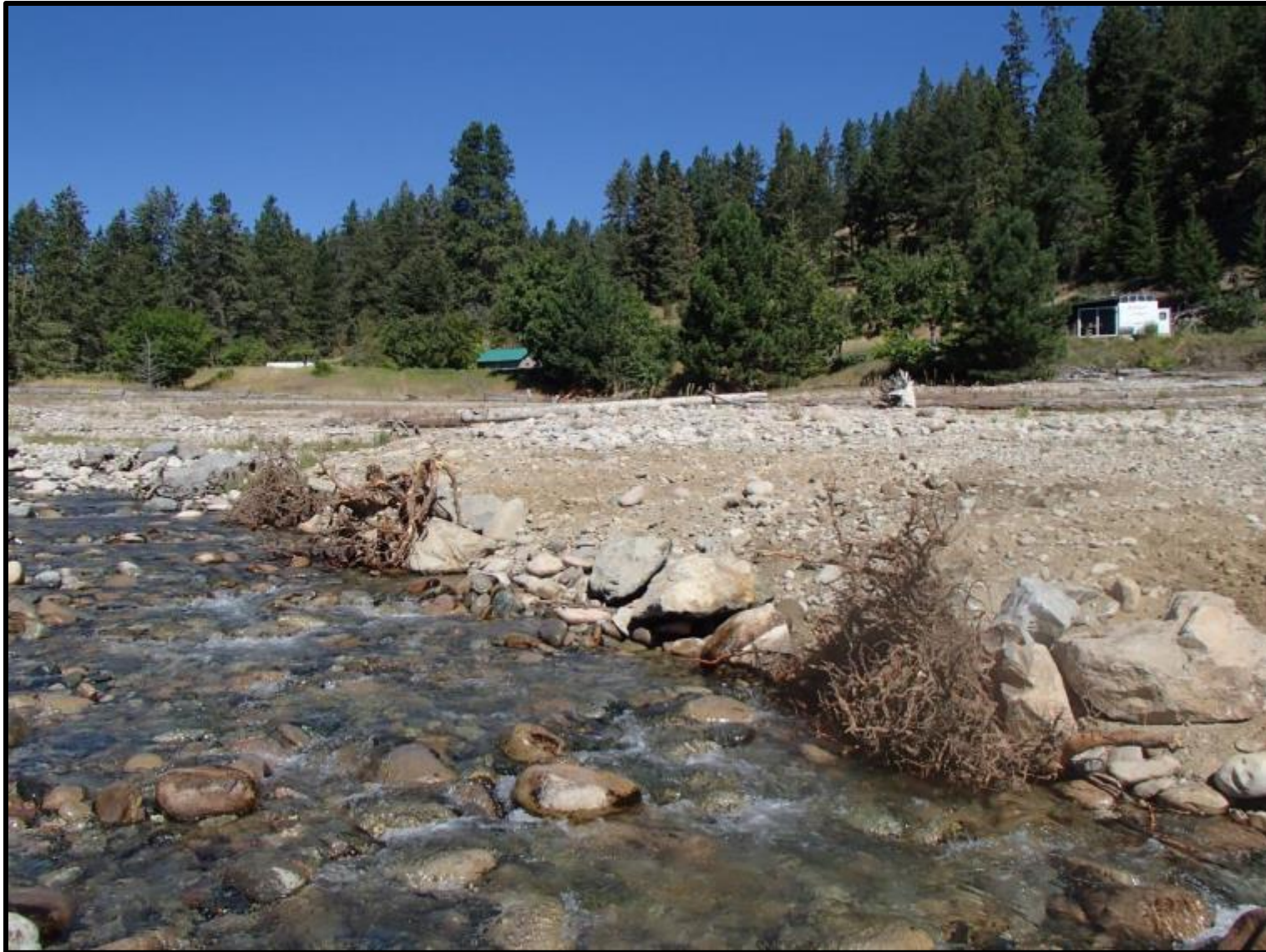
Figure 40. Structure 10 post-construction from a downstream perspective on August 12 th 2016. Photo by Evan Smith, Okanagan Nation Alliance, August 2016.
