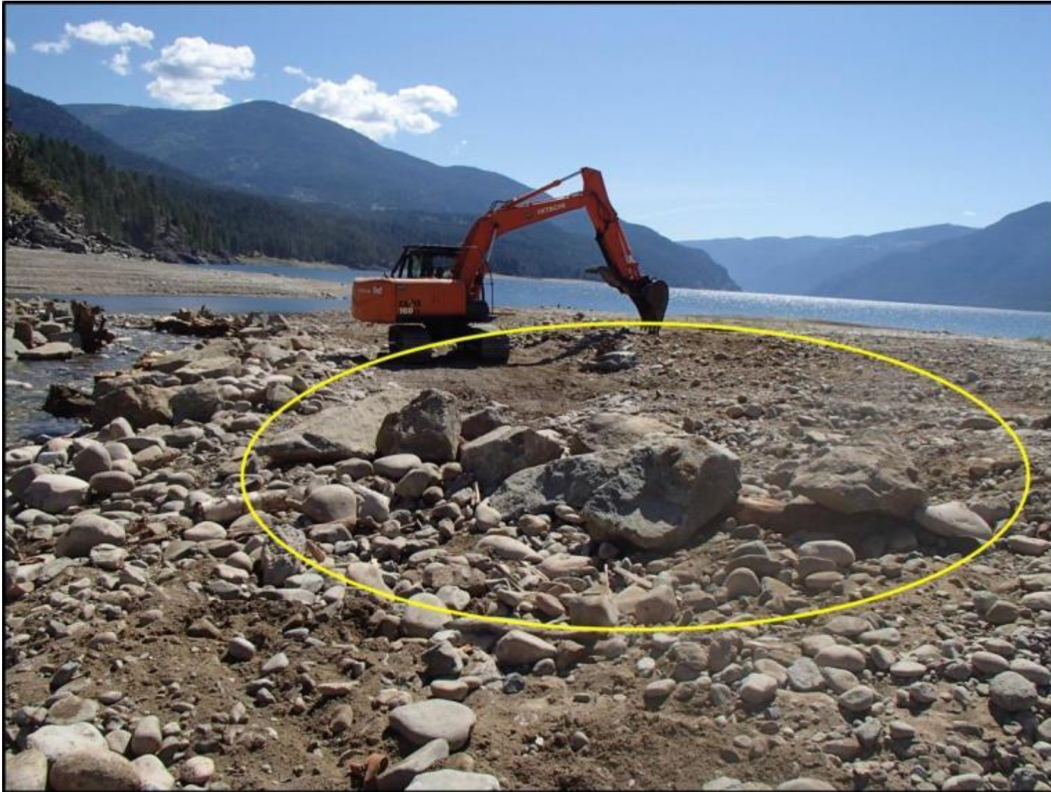
Figure 41. Structure 11 post-construction from an upstream perspective on August 12 th 2016. Photo by Evan Smith, Okanagan Nation Alliance, August 2016.
