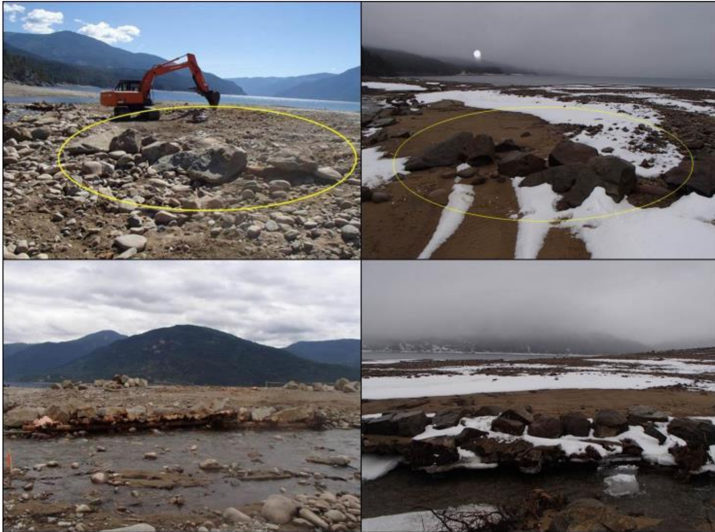
Figure 29. (Top Left) Structure 11 post -construction in August 2016; (top right) Structure 11 in March 2018 after one year of being subjected to freshet and reservoir inundation; (bottom left) Structure 12 post-construction in August 2016; (bottom right) Structure 12 in March 2018 after one year of being subjected to freshet and reservoir inundation. Photos by Evan Smith, Okanagan Nation Alliance, August 2016 and March 2018).
