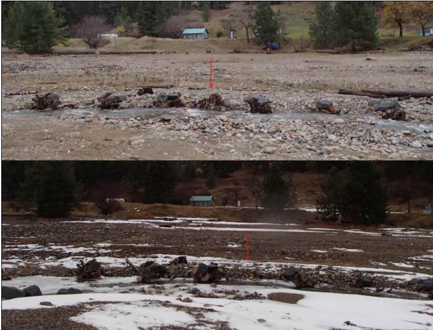
Figure 26. (Top) Structure 7 post -construction in November 2015 with a red arrow highlighting Roots 7 & 8; (bottom) Structure 7 in March 2018 after two years of being subjected to freshet and reservoir inundation with a red arrow highlighting the missing root structure consisting of Roots 7 & 8. Photos by Evan Smith, Okanagan Nation Alliance, November 2015 and March 2018).
