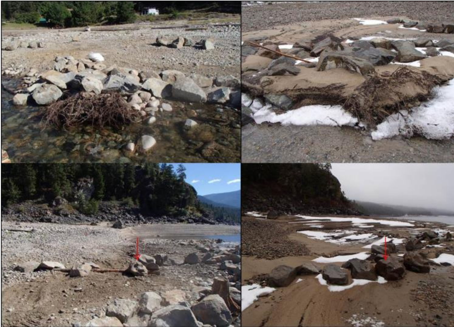
Figure 30. (Top Left) Structure 13 post -construction in August 2016; (top right) Structure 13 in March 2018 after one year of being subjected to freshet and reservoir inundation; (bottom left) Structure 14 post-construction in August 2016 highlighted with a red arrow; (bottom right) Structure 14 in March 2018 after one year of being subjected to freshet and reservoir inundation highlighted by a red arrow. Photos by Evan Smith, Okanagan Nation Alliance, August 2016 and March 2018).
