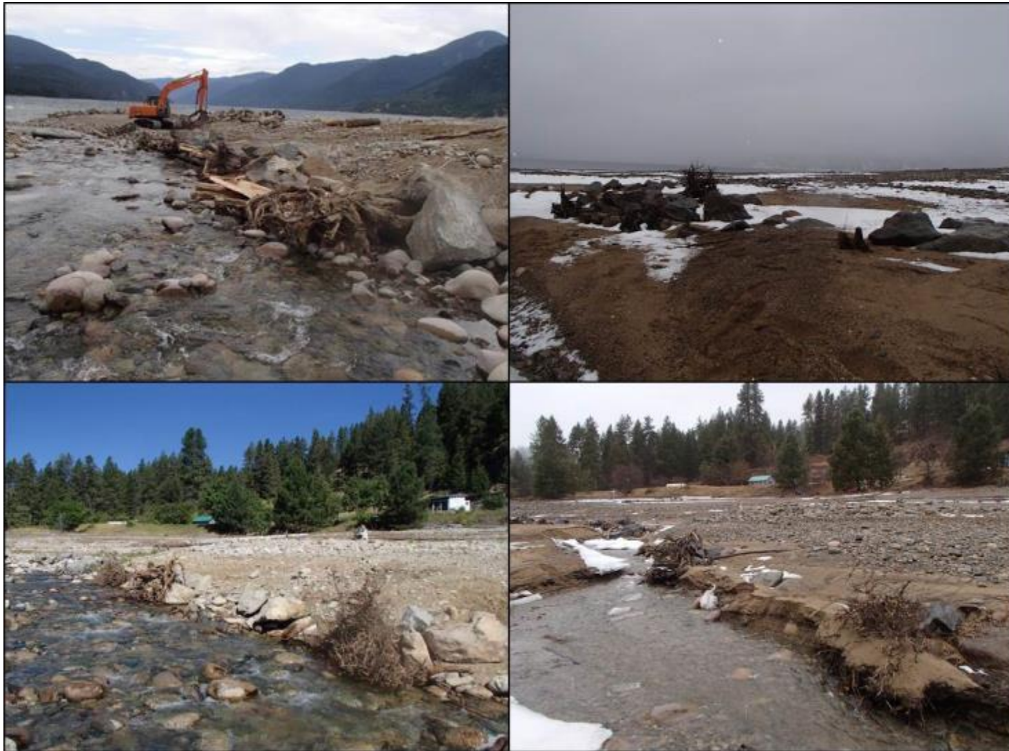
Figure 28. (Top Left) Structure 9 post -construction in August 2016; (top right) Structure 9 in March 2018 after one year of being subjected to freshet and reservoir inundation: note the amount of sediment deposition on top of the structure; (bottom left) Structure 10 post-construction in August 2016; (bottom right) Structure 10 in March 2018 after one year of being subjected to freshet and reservoir inundation. Photos by Evan Smith, Okanagan Nation Alliance, August 2016 and March 2018).
