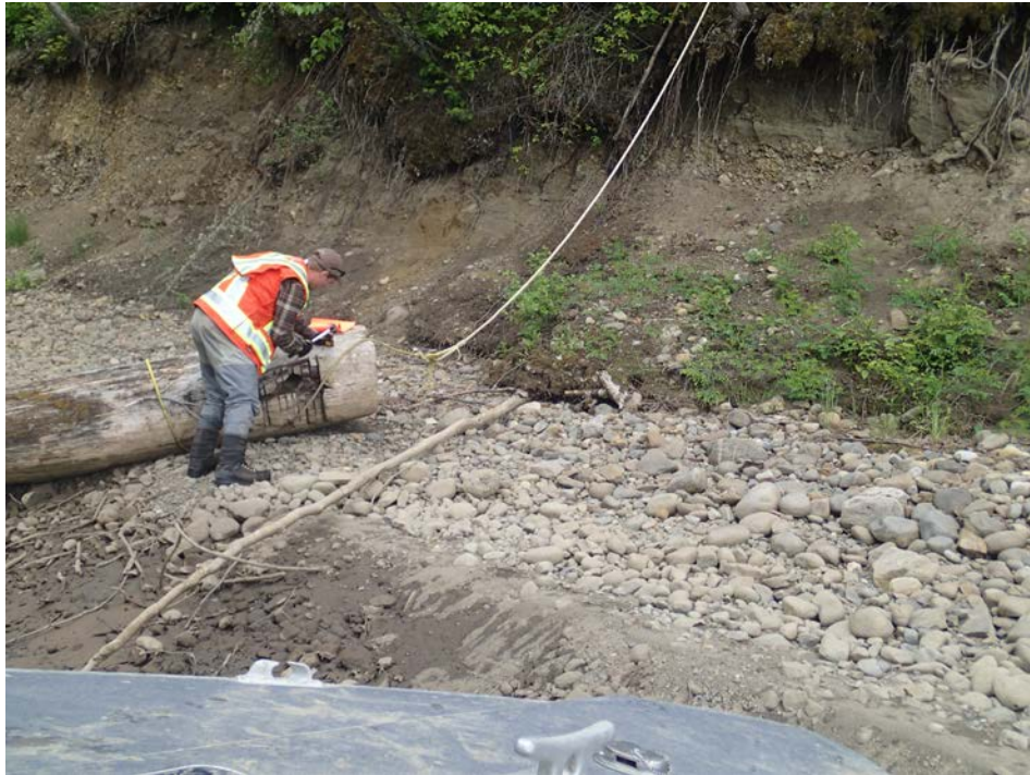
Site 5: Another example where cable clamps rust out and structure is free which can become a boating hazard.
