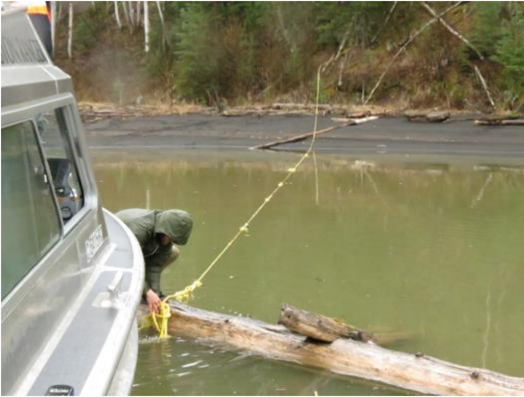
Site 3 boom: boom is resecured to land with poly rope.
