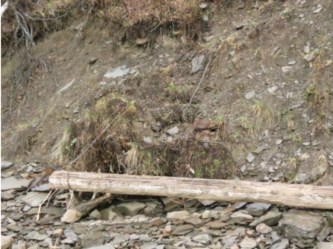
Site 2a: earth anchor in place but land has slumped.
