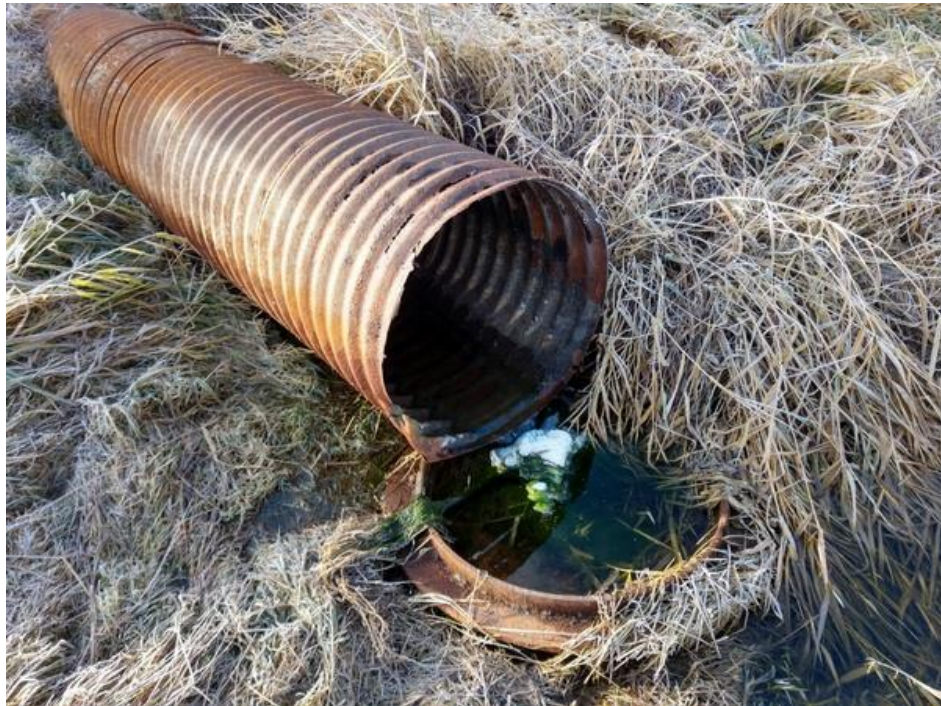
The entire KUPI Marsh Impoundment was designed to be drained by this culvert. The gate on the culvert is broken, and the culvert is rusted. The culvert is temporarily blocked with mud and a stump. The culvert may be permanently blocked in a future restoration project.
