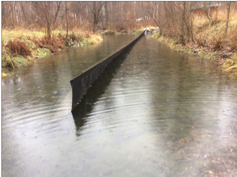
Photo 2. View SW of the settling pond. Note the shoreline of the pond, which provides easy access for the tracked excavator used in the removal of the pond sediment.
