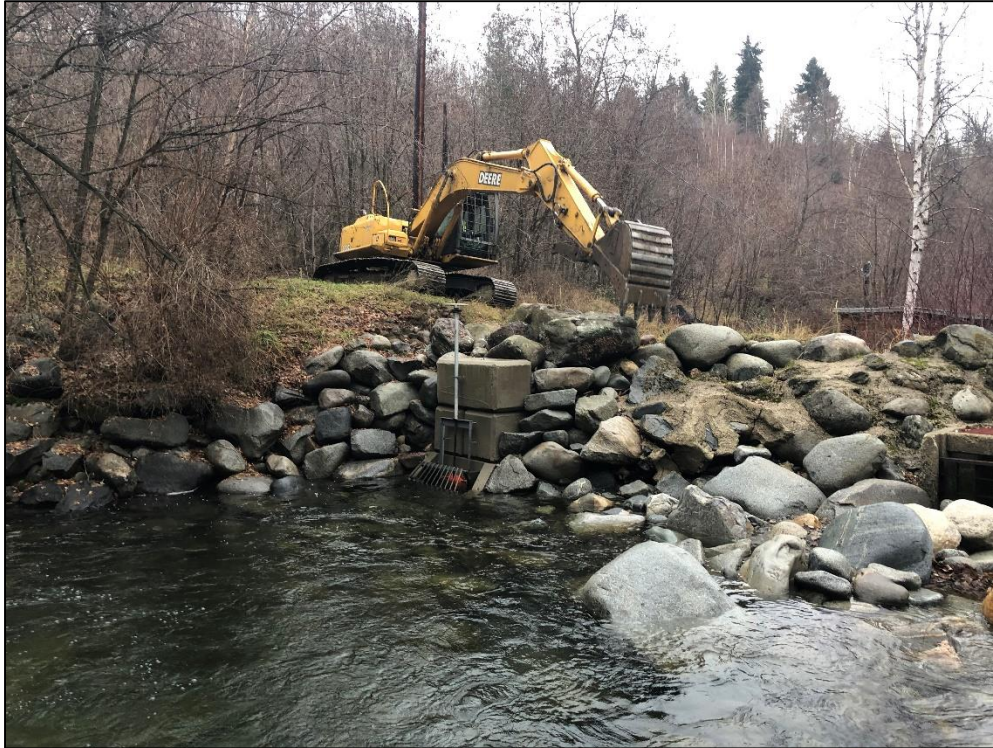
Figure 11: Placing boulders around and on top of the intake barrier wall to increase armoring.
