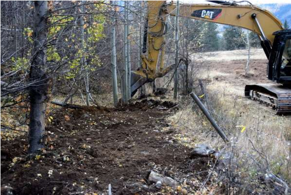
Photo 17: A section of a former ditch is being filled and brought to grade
