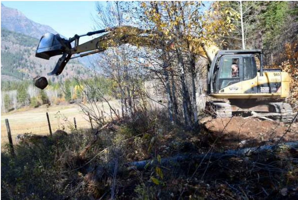
Photo 12: The excavator gathers boulders from the edge of the hayfield to be used to create unique habitat features along the creek and wetlands
