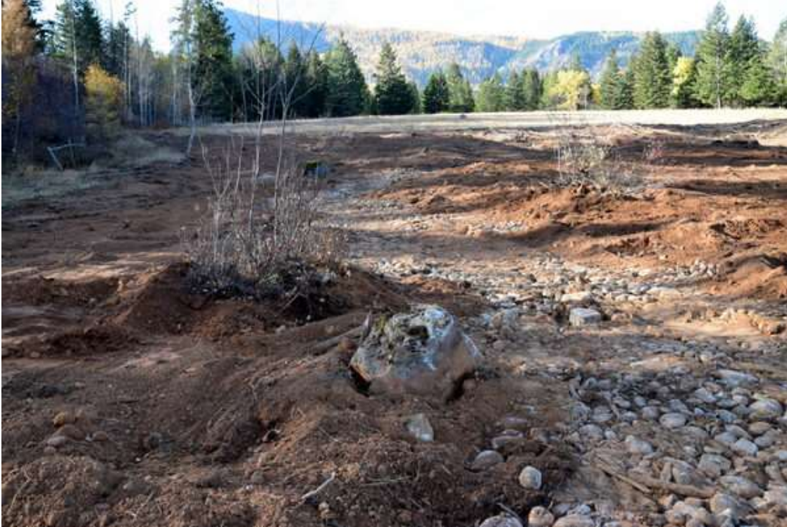
Photo 28: Restored creek and floodplain, looking downslope. Note the boulder placement and re-planting of shrubs in the foreground and background
