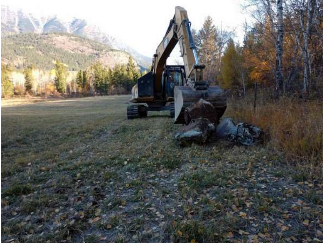
Photo 13: Here large boulders are being gathered for use in the restored stream
