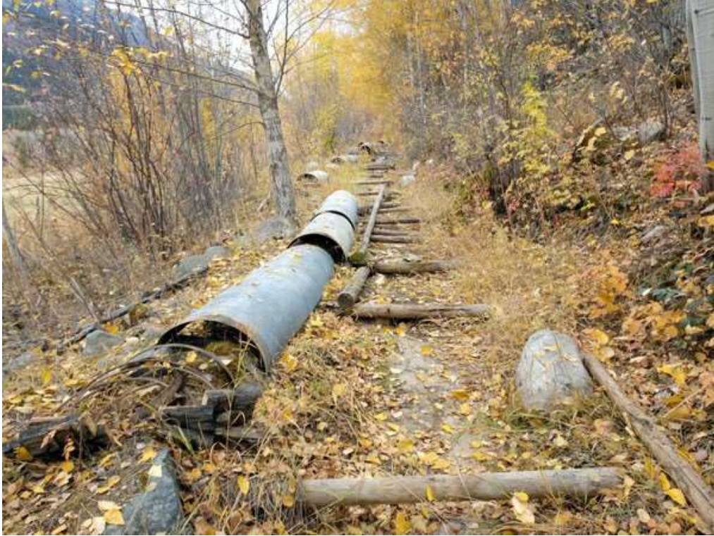
Photo 3: Part of the project involved removal of a metal flume used to divert Douglas Creek
