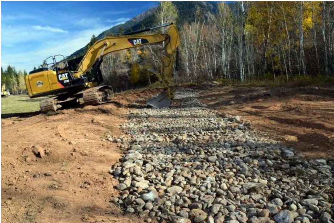
Photo 8: Small rock was used to armour steeper sections of the restored creek. The rock was covered with a thin layer of soil so it could be seeded
