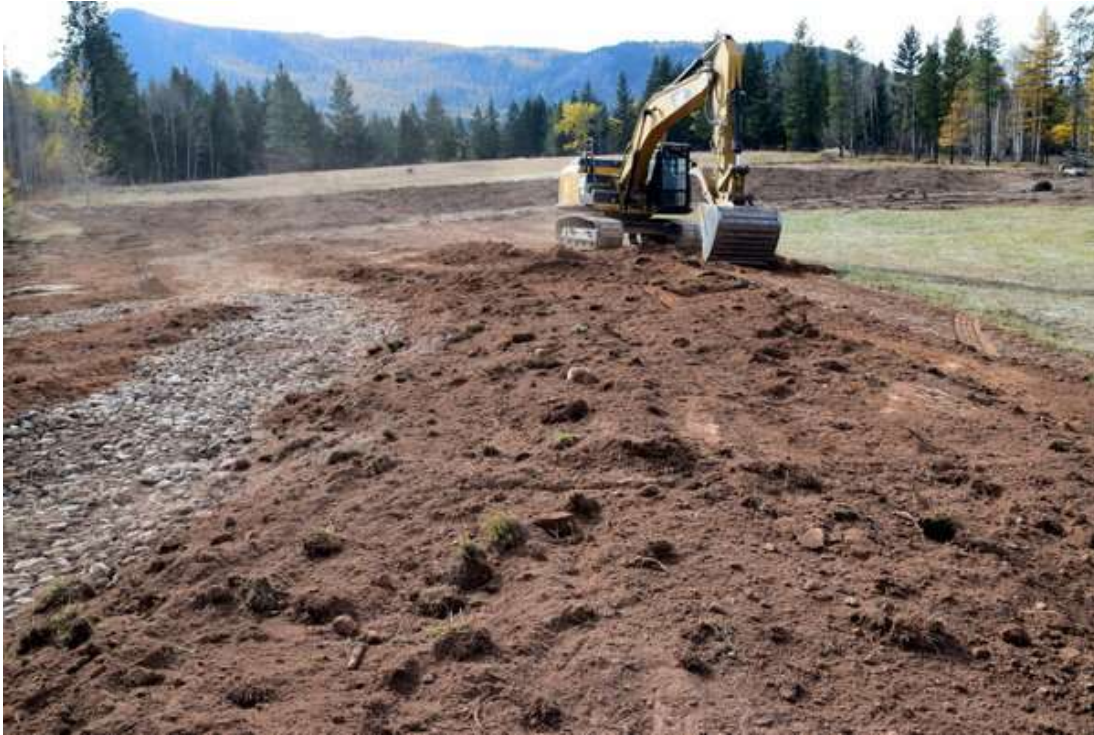
Photo 11: The excavator shapes low banks with gradual slopes and loosens compacted soils on the restored floodplain.
