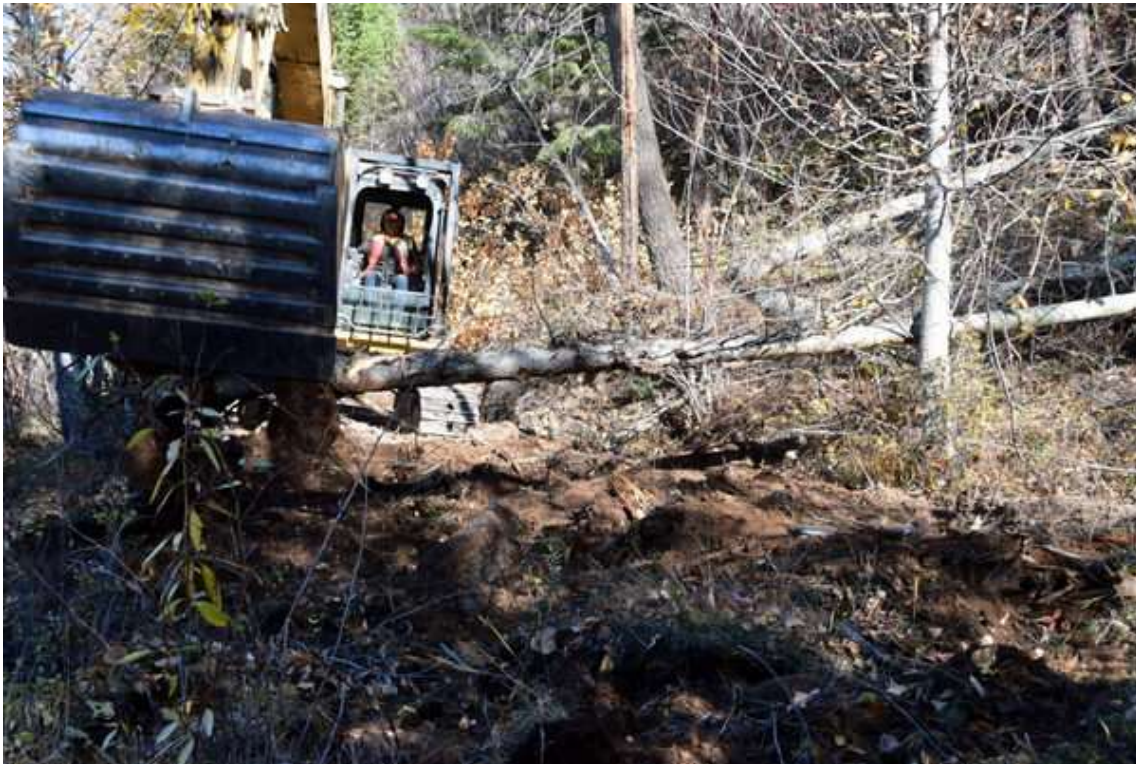
Photo 16: The excavator is used to fill and naturalize the ditches, as part of the overall project, thereby ensuring that flows from Douglas Creek would not be lost
