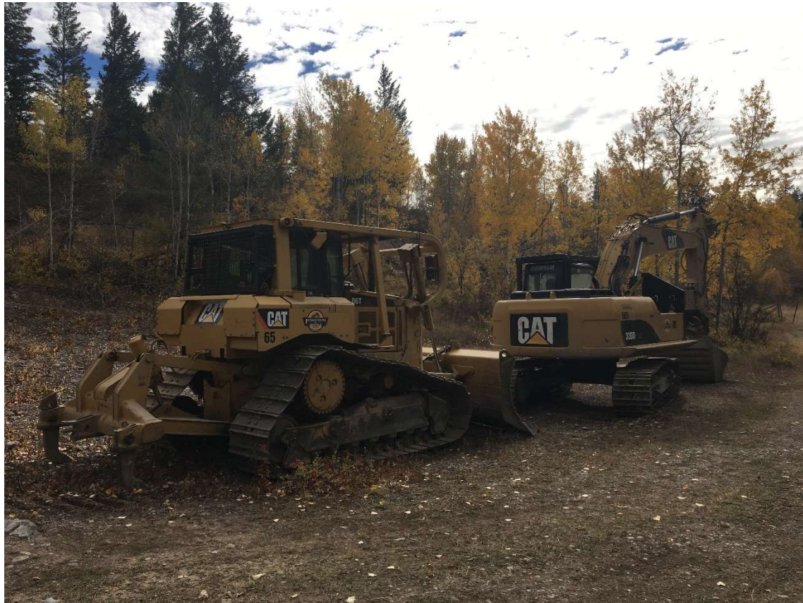
Photo 33: Two excavators, a dozer, a dump truck and a tractor were used on the project
