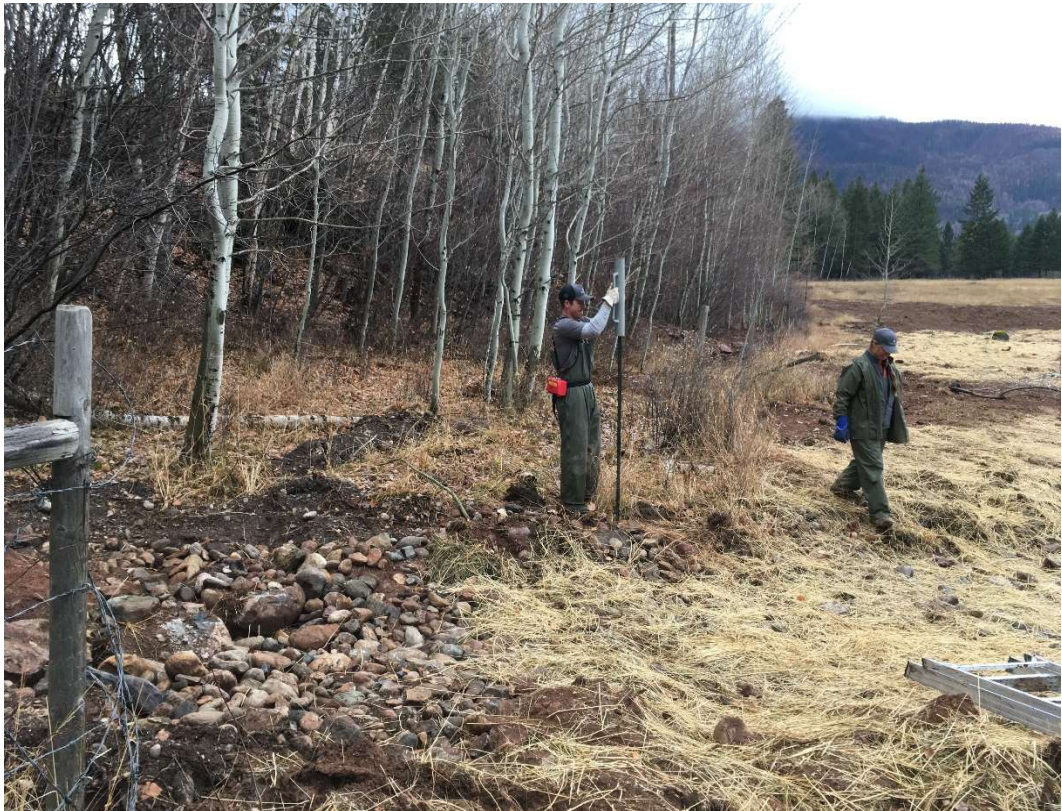
Photo 35: Fences were re-built following earthworks to keep livestock out of the site
