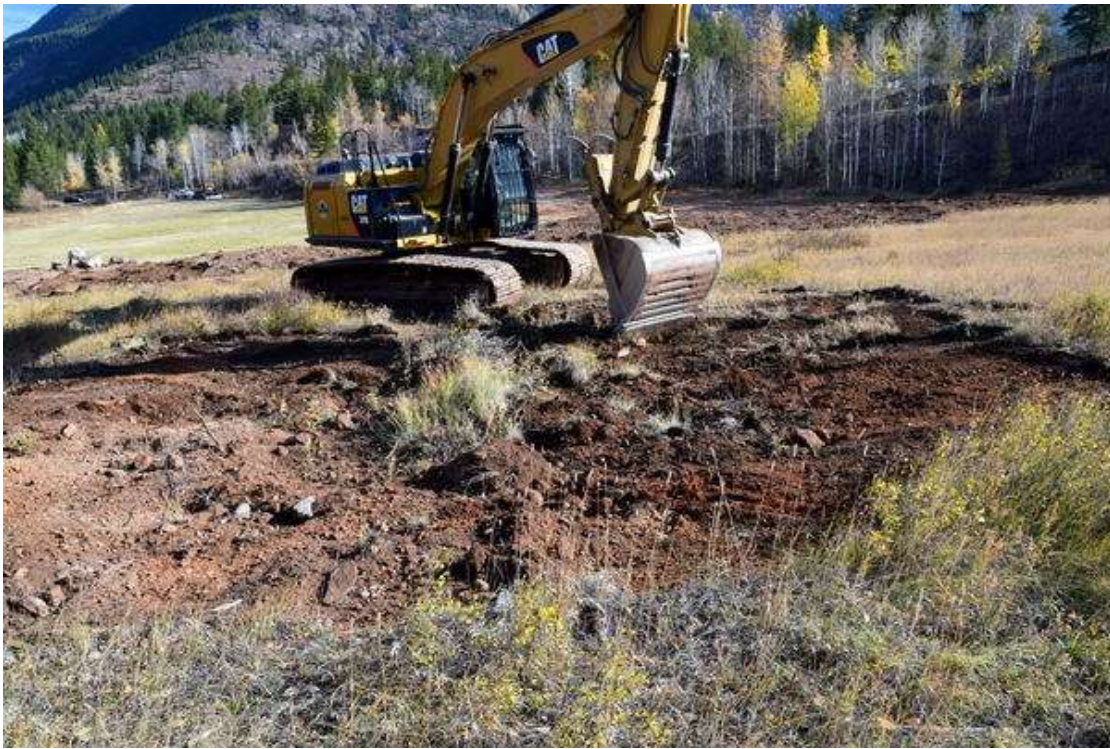
Photo 21: Here a small borrow pit from years ago is being restored, beside the restored creek
