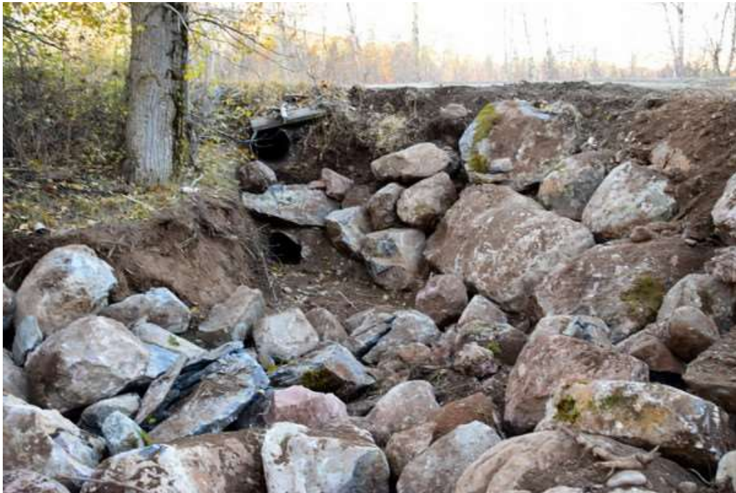
Photo 20: This photo shows the two culverts carrying water from Douglas Creek under the Bull River Forest Service Road. The culverts were unplugged during the project, and erosion was controlled by placing rock salvaged alongside the FSR
