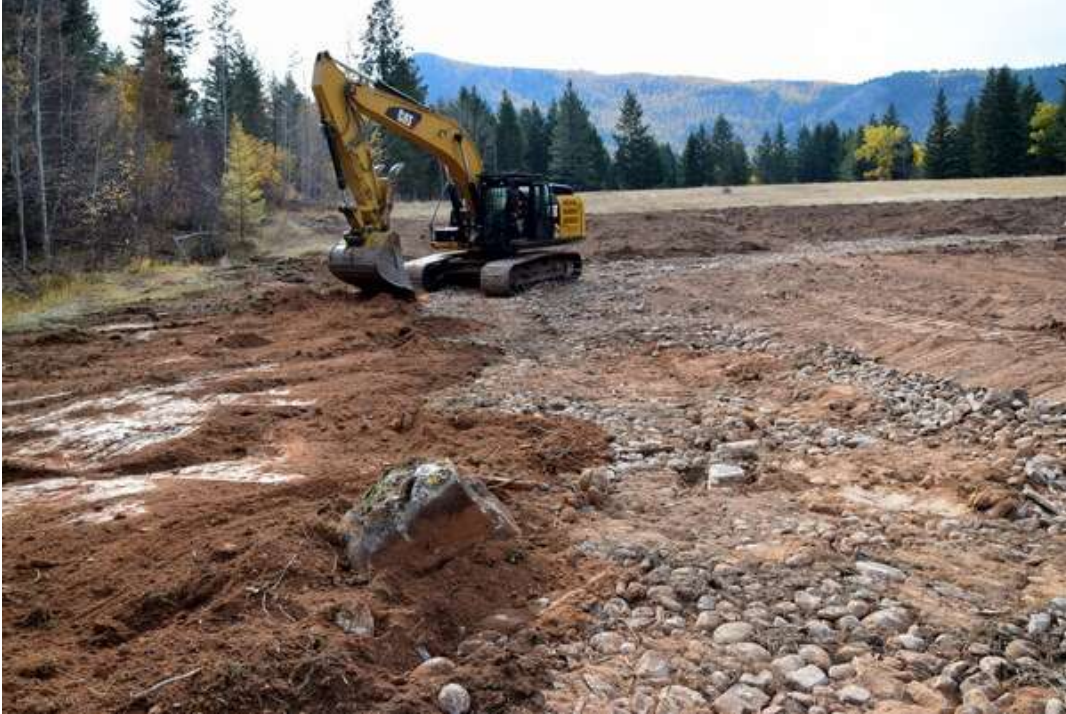
Photo 9: Soil is spread over the rock so the restored floodplain will support a diversity of sedges and rushes without erosion and appear more natural looking within the site context
