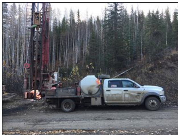
Drill rig setting up to drill OW482, Fort Nelson BC. Photo: J. Yin.
