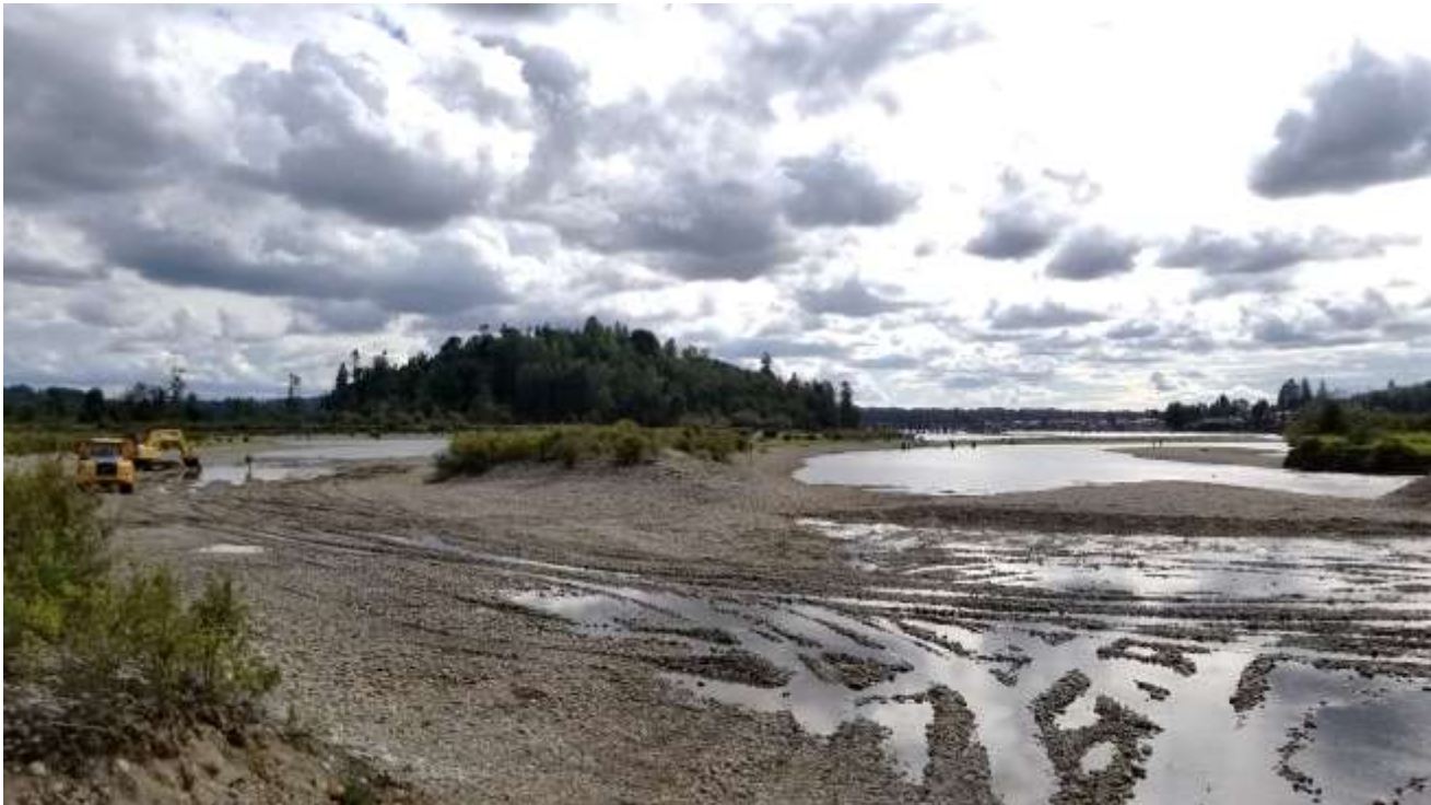
Figure 3. South-view, downstream of project site showing (left) dry channel 5 and channel 4 with the elevation drop, during construction.
