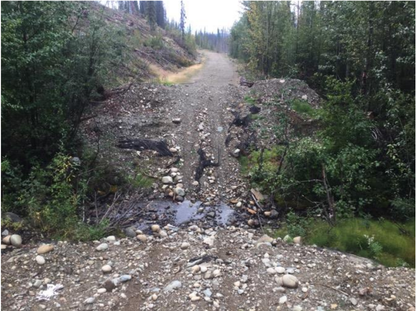
Figure 26. Road to Tutizzi Lake ditched to prevent pickup truck access.
