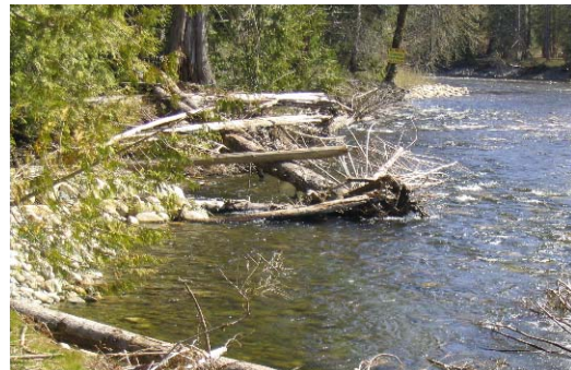
Photo 14. Looking downstream at site 7+120 further modified in 2004 to capture debris.
