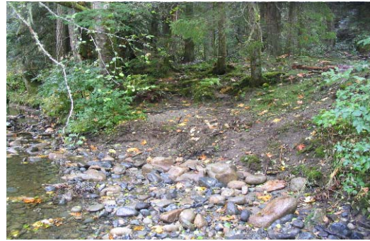
Photo 2. Looking at lowermost access near 3+800 after deactivation.
