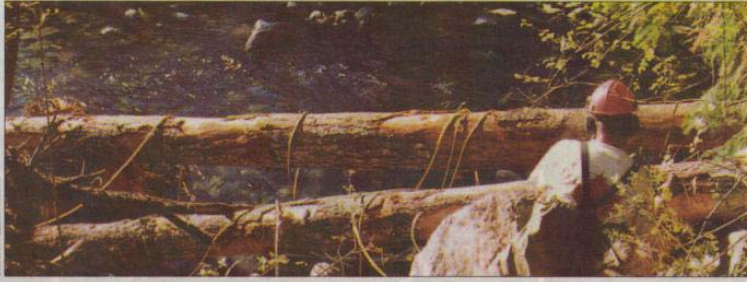
CREWS WERE WORKING at using cables to secure the large logs and rocks that make up one of the four new Large Woody Debris structures along the Little Qualicum River Friday morning.
