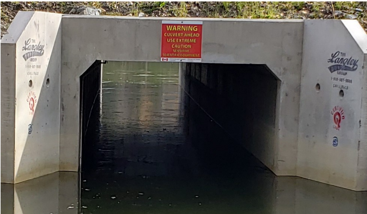
Signage warning water sport users to use caution if moving through culvert (signage installed at both sides of the culvert)
