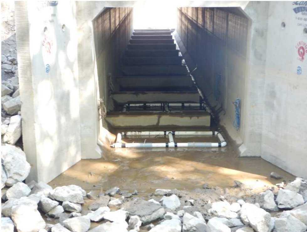
Figure 3: A new 3m x 3m box culvert was installed in May of 2019 providing improved access to juvenile salmonids between the river and the estuary. Note acoustic arrays (for Instream fish monitoring study in 2019) and gap in concrete baffles to right to allow fish passage.
