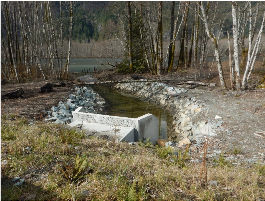
March 15, 2020. Facing west from Training Berm (towards Squamish River intake); note placement of additional rip rap along banks leading towards river to provide erosion protection
