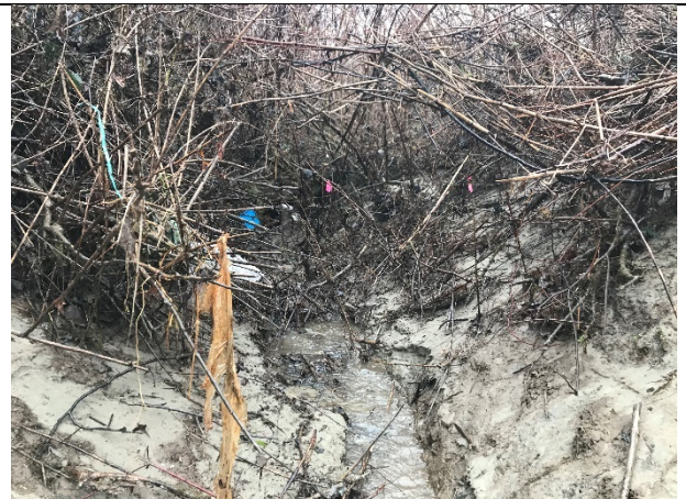
Photograph 7 – Upstream view of nominal drainage function through recently deposited floodplain sand veneer following February peak flows.
