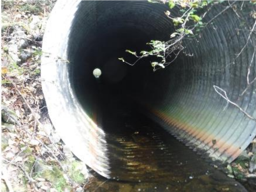
Figure 78: Railway crossing (modeled crossing 16603287) located 200 m upstream of PSCIS crossing 125247 (UTM: 10N 542901 6062899).
