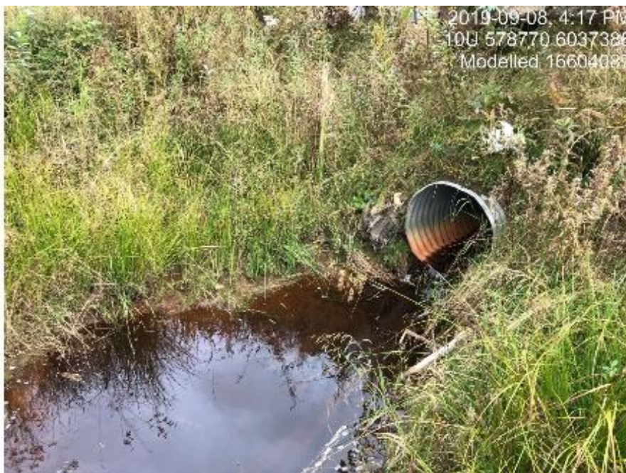
Figure 38: View of crossing 16604087 - located on small tributary upstream of PSCIS crossing 125000 (UTM: 10N 578771 6037388).
