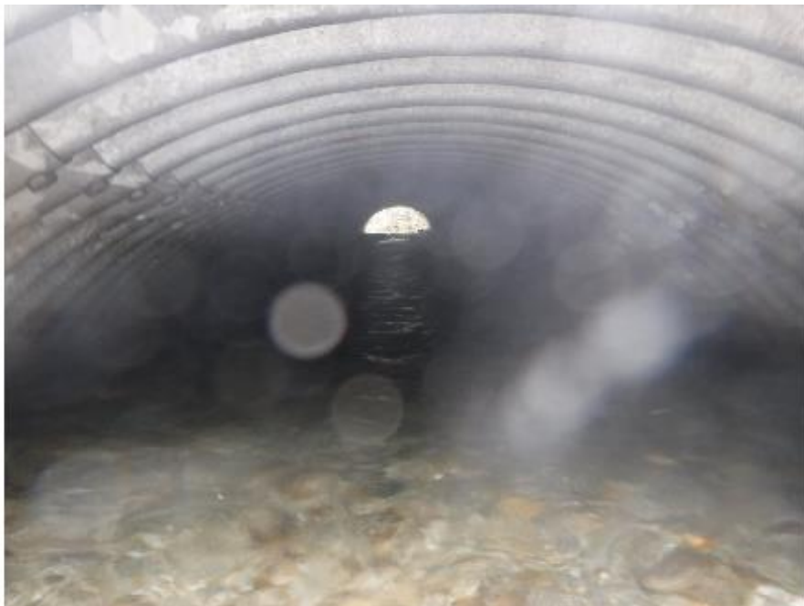
Figure 70: Passable railway culvert (modeled crossing 16603278) located downstream of PSCIS crossing 125231 (UTM: 10N 549788 6065094).
