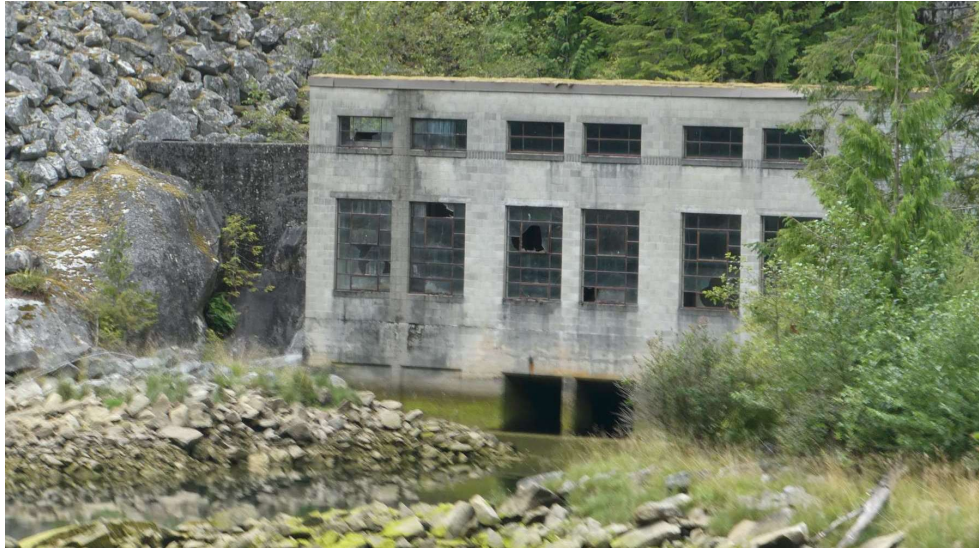
Figure 13. The Auxiliary Building contains substantial bat guano.
