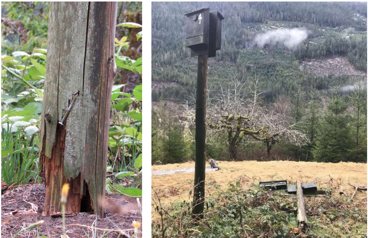
Figure 2. Rotten Post Supporting Clowhom Maternity Box Cluster.
