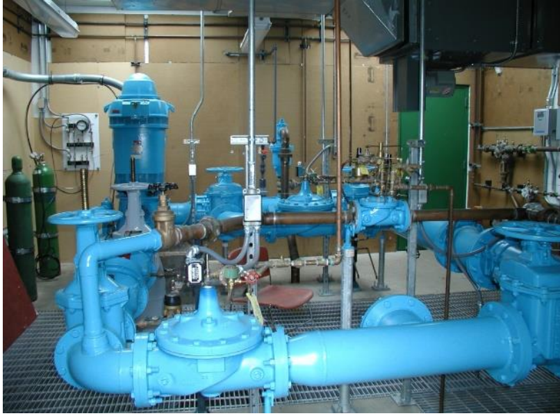
Figure 5: Pump house interior view of ASR wellhead – Beaverton, Oregon (USA). Source: GSI Water Solutions.
