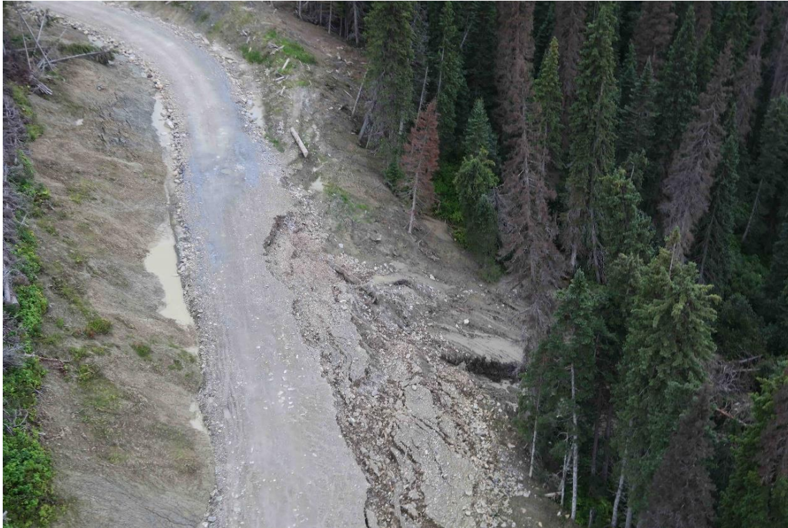
Figure 13. Slumping of newly-constructed forestry road into Anzac River floodplain at stream km 48 (10 U 553116 6093016).
