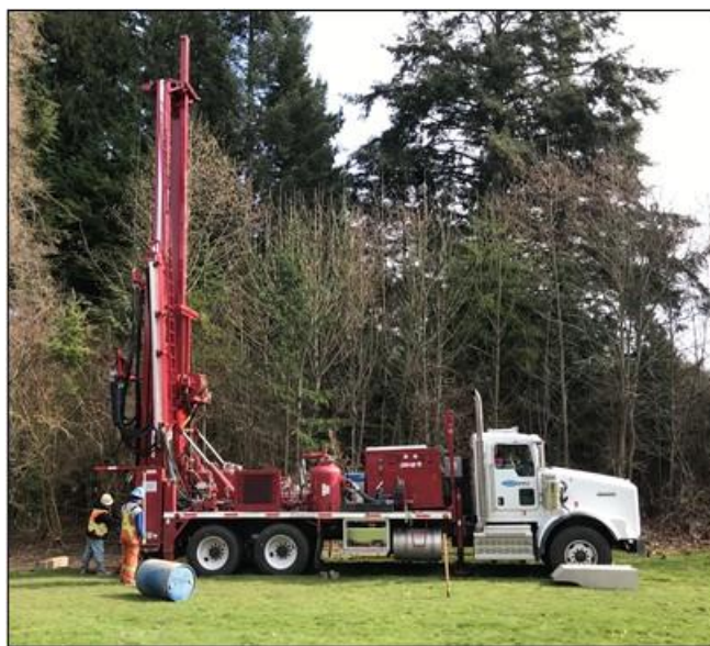
Drilling of OW498 with rotary drill rig in Mission Point Park, Sechelt.
