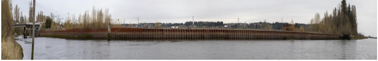
Figure 4: Panorama of the 440m steel clad retaining wall that separates the current site from Courtenay River.
