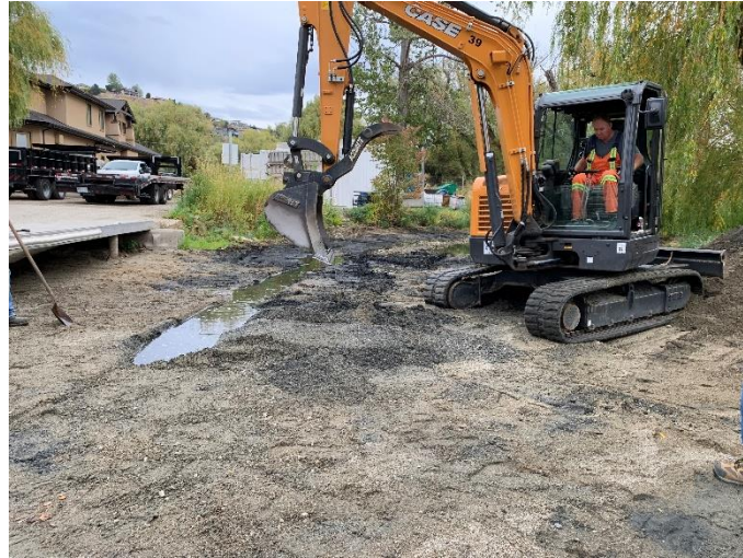
Photo 3 – A small excavator walked out onto the sediment bar and removed the sediment from the south side of the work area
