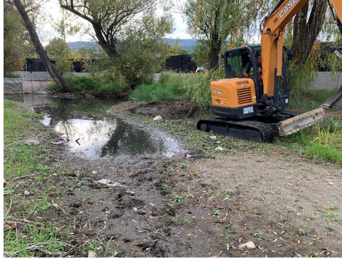
Photo 5 - The dredged area extended outside of the proposed dredging area because of the extent of sediment
