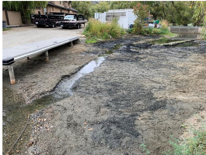
Photo 4 - Excavator dredged out sediment in the work area leaving a 0.4 m wide trench from the base of the lagoon to the lake
