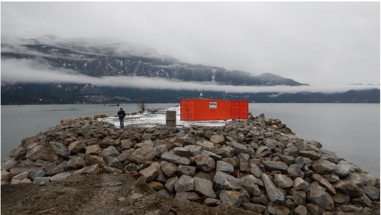
February 3, 2022. Armour placement at north end of Spit Island completed. Facing south.
