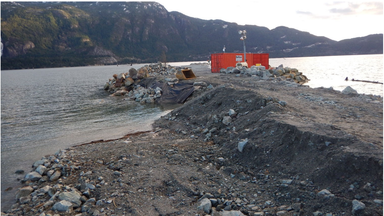
January 31, 2022. No construction during high tide. Note placement of geofabric beneath newly placed armour rock
