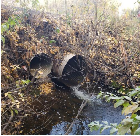
Photo 1. Perched culverts at Dog Creek FSR.
