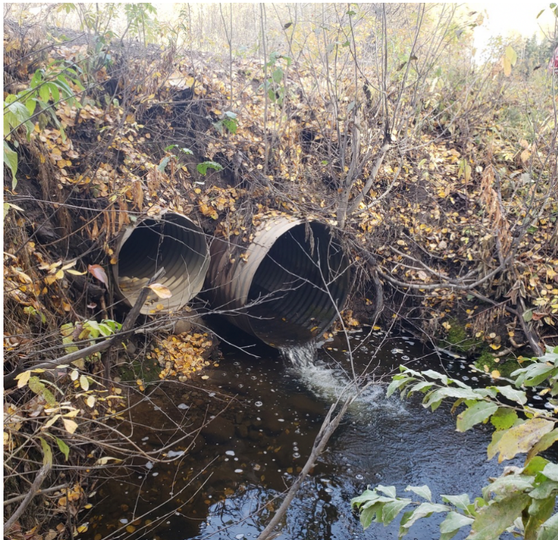
Photo 1. Perched culverts at Dog Creek FSR. Photo by Barry Booth
