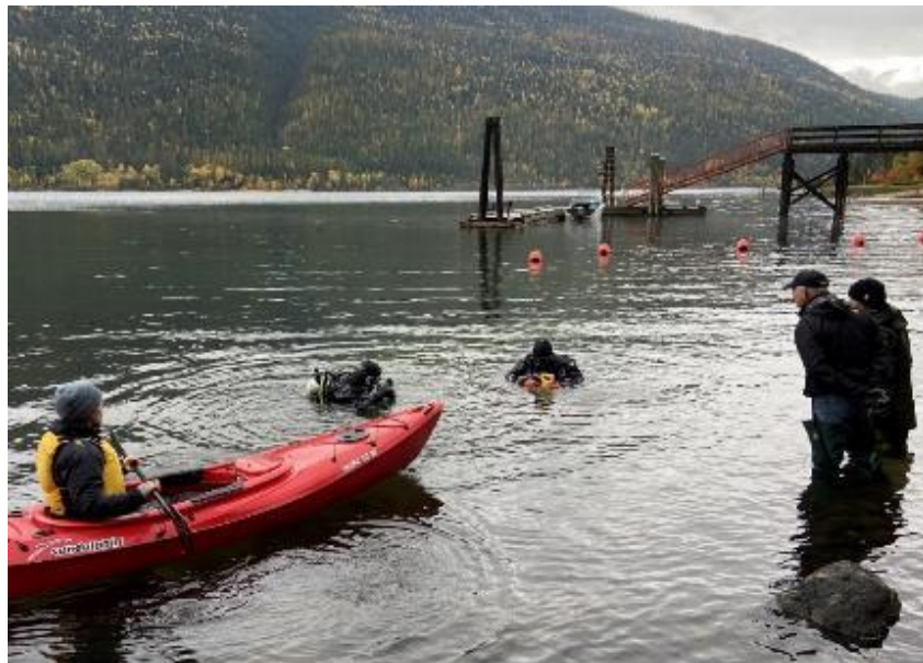
Figure 4: Oct 28, 2022, Kokanee egg capsule install. Divers installing egg capsules. Photo credit: Moriah Tanguay
