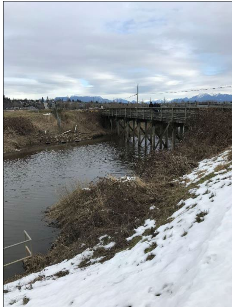
Photo 4. Looking upstream at the 168 Street bridge crossing over the Serpentine River on February 27, 2019.
