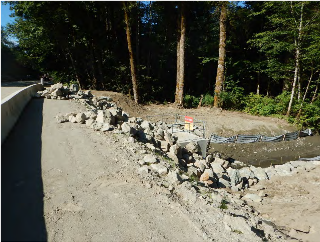
Photo of stockpiled material on south quadrant of west side of Culvert #2
