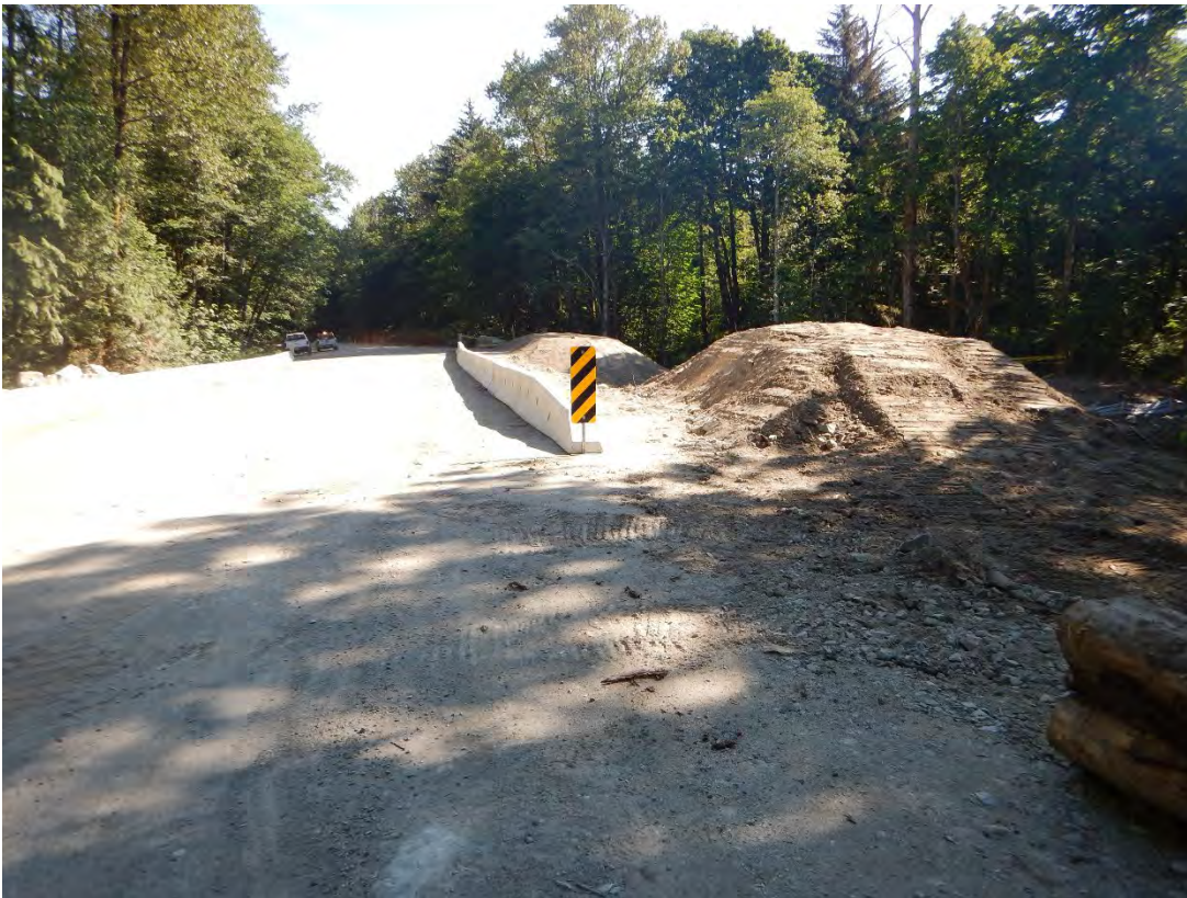
Stockpiles on north and east side of Culvert #2 on estuary side (east side of road)
