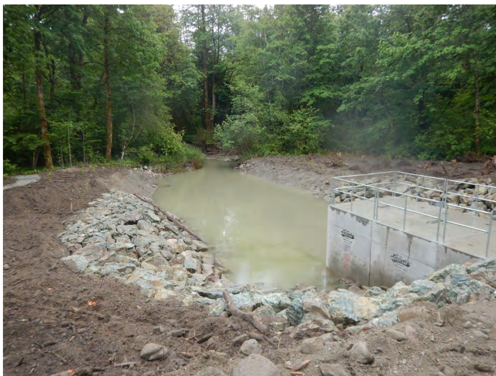
Facing east towards central estuary – note organic placement on each side of culvert
