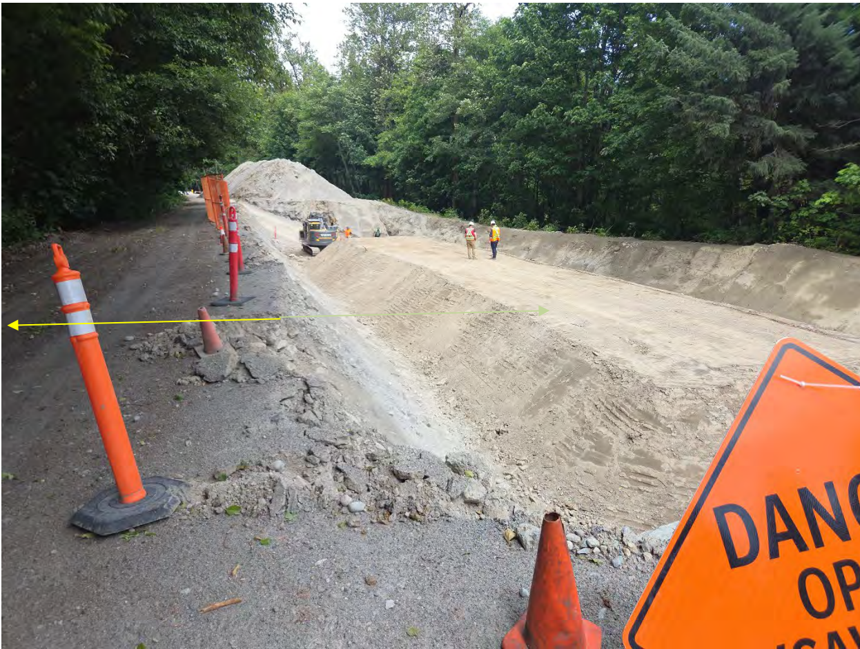
Photo 2. Placement of JK impacted fill complete. Note the western slope extends into the “road”. The dimensions of the stockpiled contaminated soil were approximately 35m in length, 6-7m in width (wider at the base), and 2m in depth.
