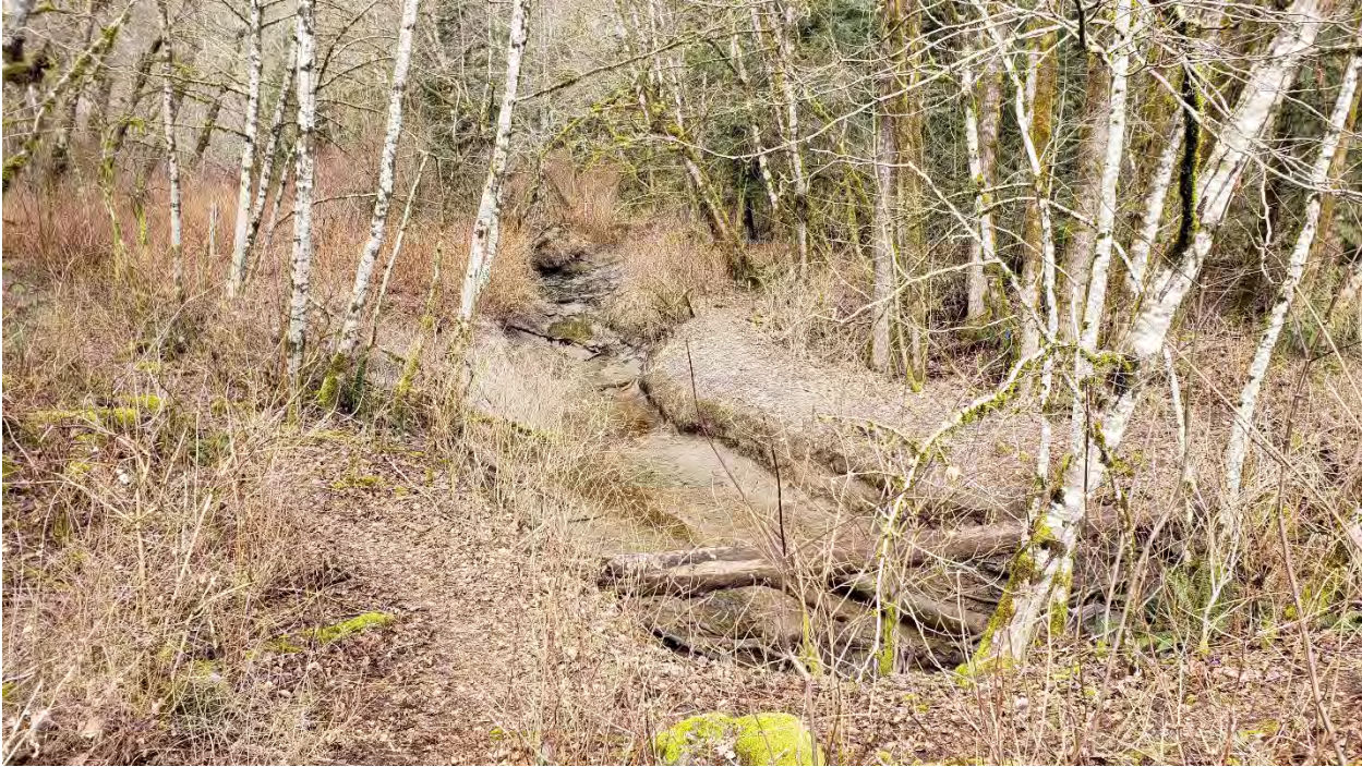
West side facing towards river from top of Training Berm (note culverts are buried behind debris)
