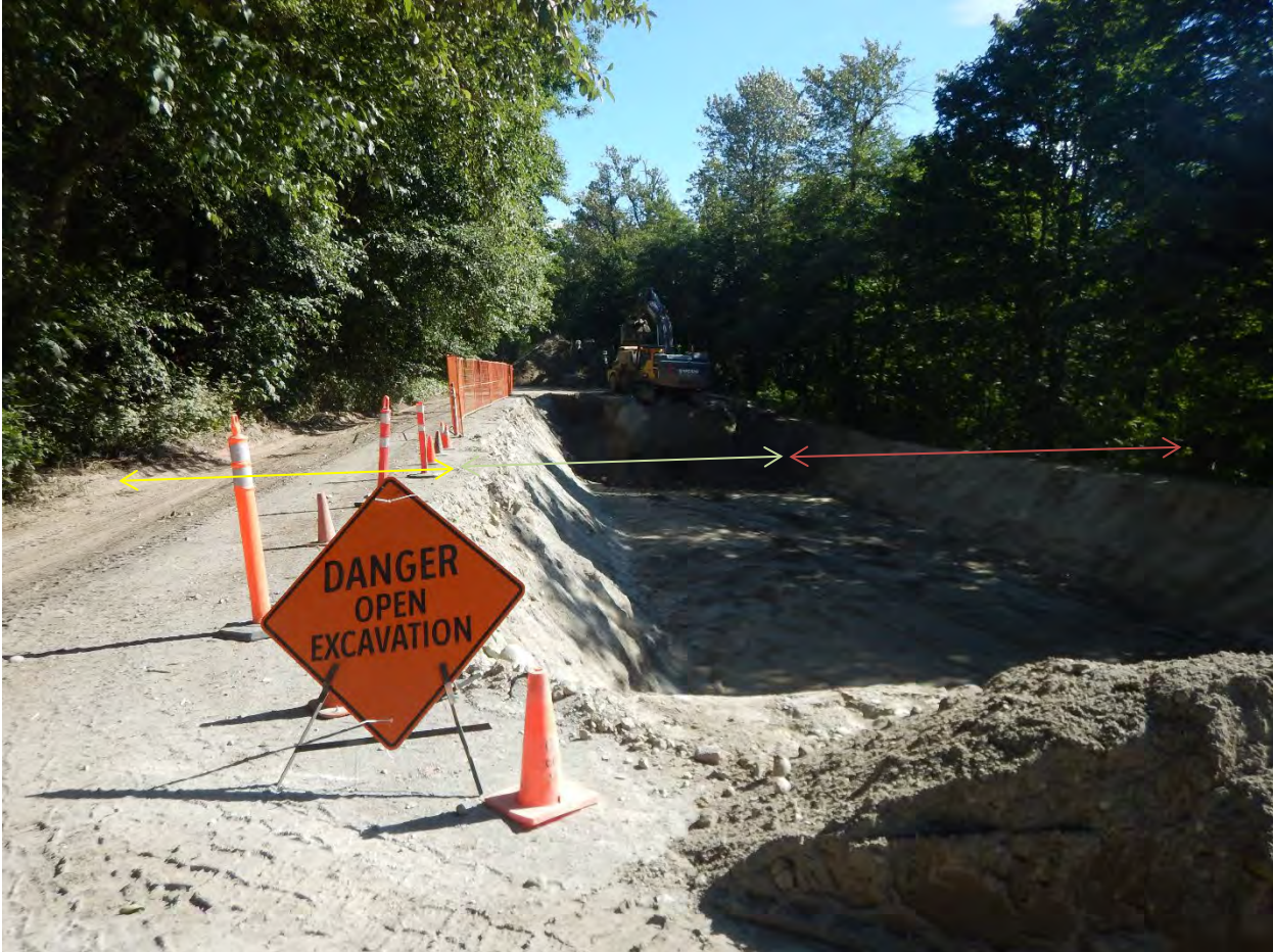
Photo 1. Approximate width of road depicted with yellow representing west lane of Berm/Spit Road and green representing east side. Orange line depicts approximate width of east shoulder. Pit dimensions approximately 13m in width at the surface and 8m at the base, 50m in length and the depth was 4m.
