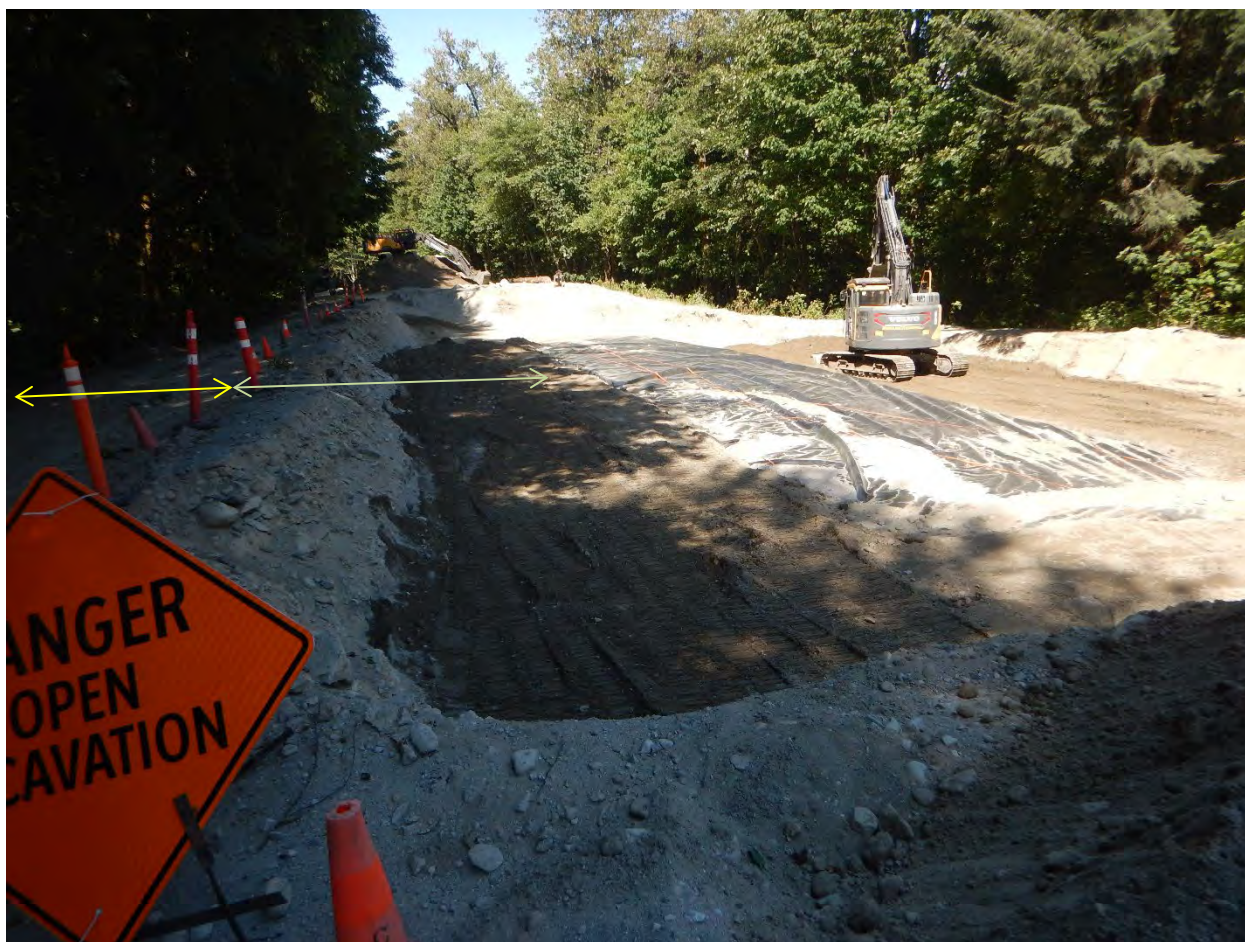
Photo 4. Backfilling underway, note ribbons of “invasive species” flagging tape placed along top of liner and every metre until top of berm as warning for any future disturbance.
