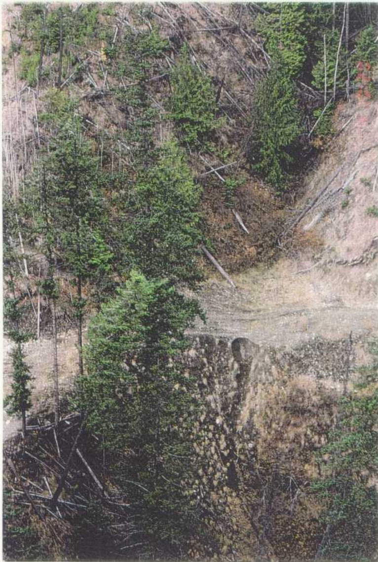
Photo 11. FE7, TP13. No culvert at gully crossing. Water across road initiating fillslope failure.
