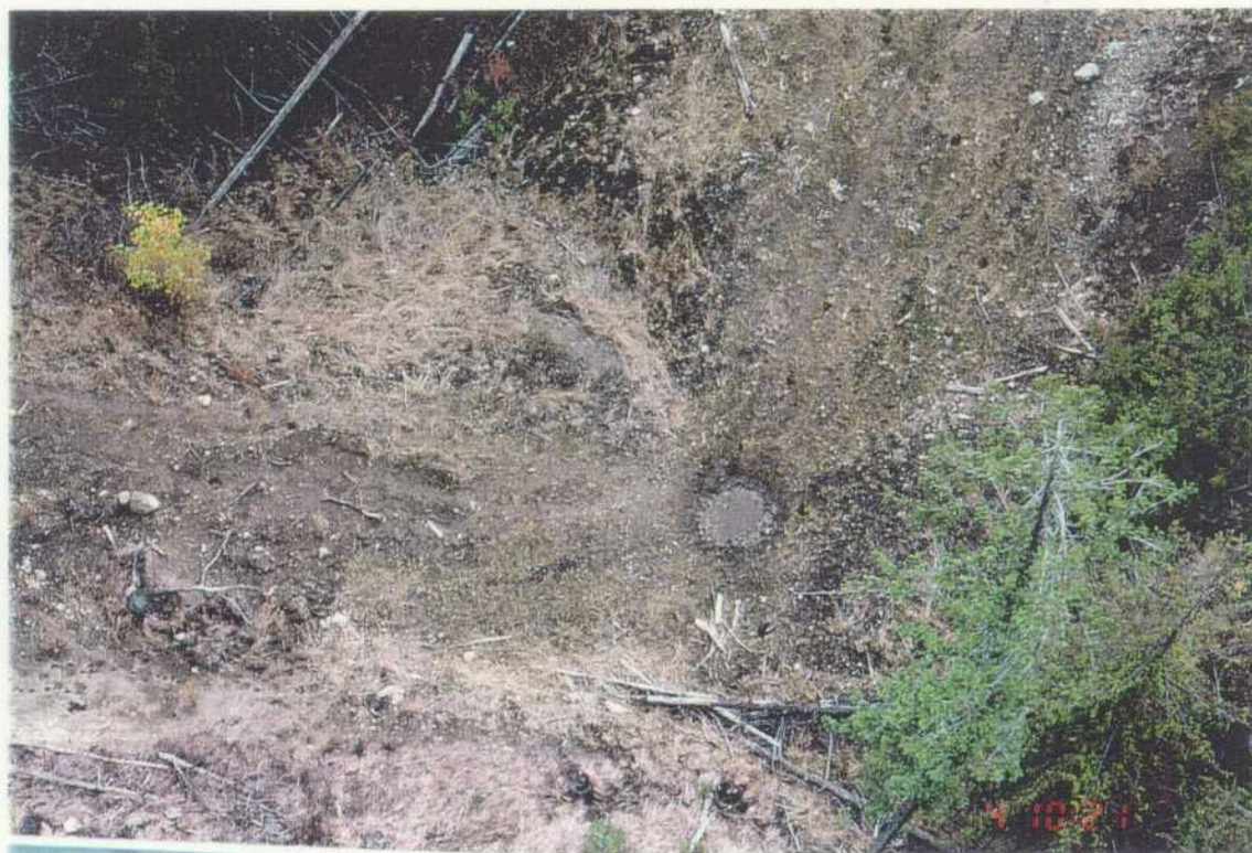
Photo 10. FE7, TP12. No culvert at gully crossing. Water and sediment crossing the road. Potential for failure below the road (see Photo 11).
