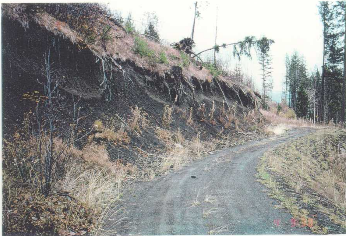
Photo 7. FE4, Section 2. Sloughed cutslope. No functioning ditch. Blocked culverts intakes.
