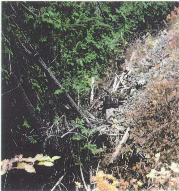
Photo 8. FE4. Fillslope supported by organics and trees, on 80% sideslopes of gully connected to Reach 7 of Ferry Creek (see Photo 9).
