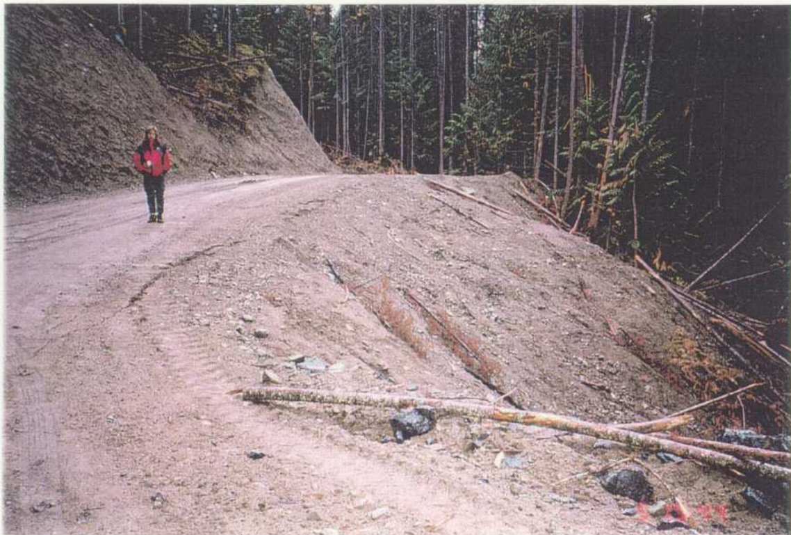
Photo 16. FE6, TP48. Long tension crack in large fill leading into ephemeral gully.
