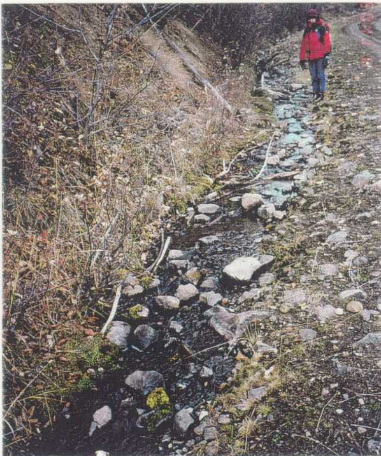
Photo 14. BS, TP14. Creek flow diverted down ditchline. Run-out on flat bench.
