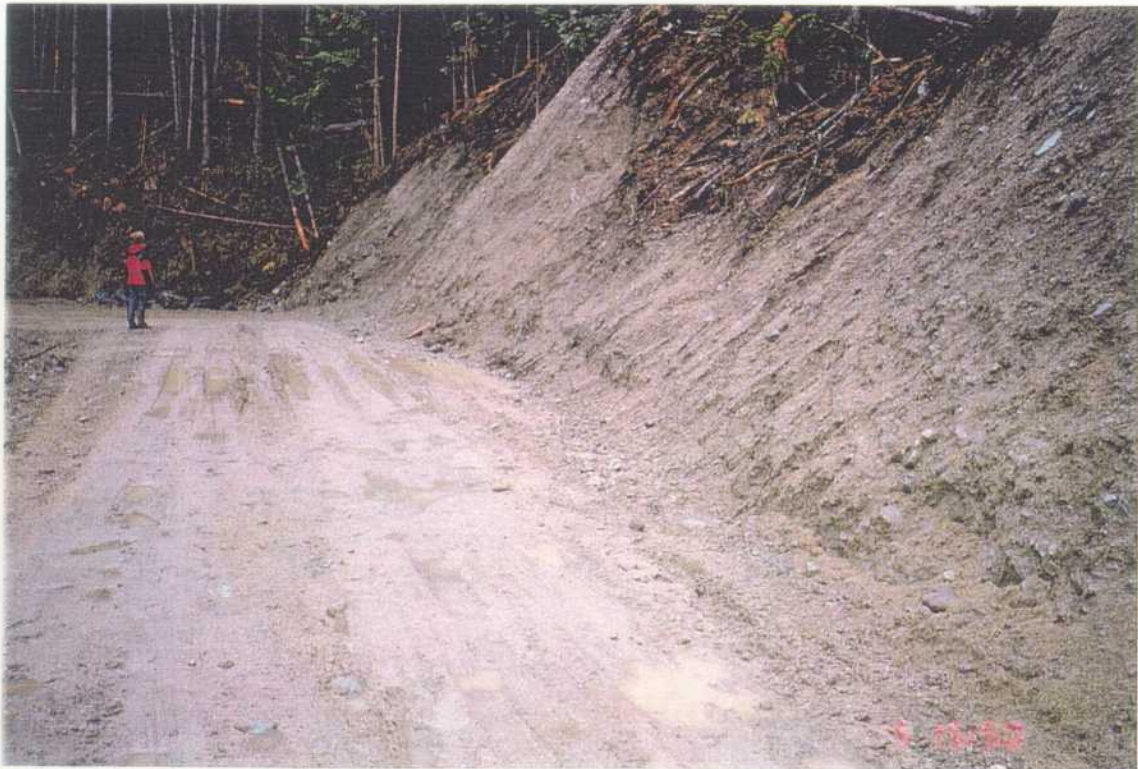
Photo 15. FE6, TP48. Sloughing cutslope, no functioning ditch. Low road grade crossing gully sidewalls. Water draining to fillslope – see Photo 16.
