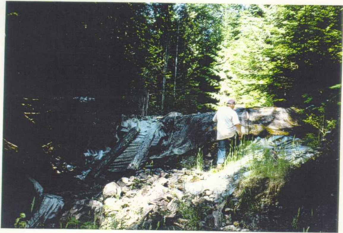
Photo 3 – Washed out water diversion structure on Halley Creek (June, 2000)
