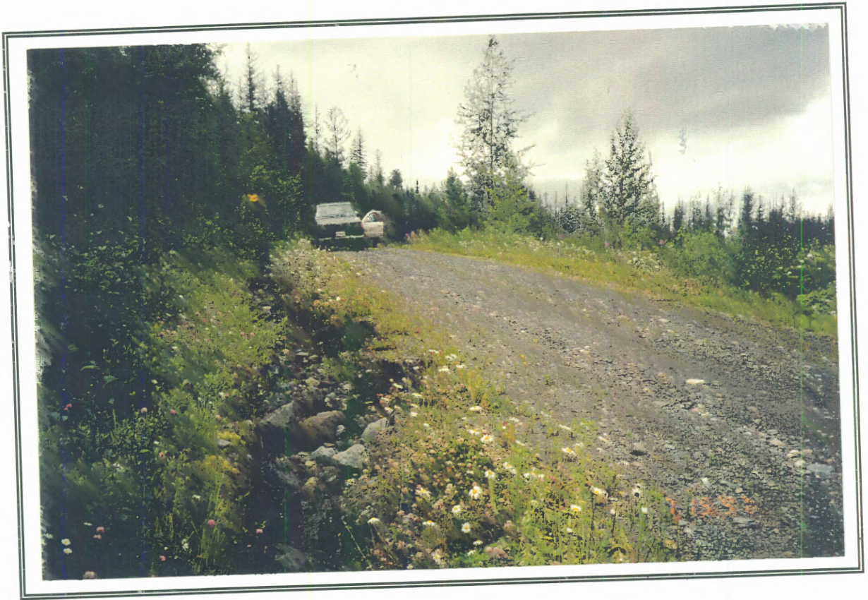
PHOTO MCKIN12. Ditch erosion resulting from infrequent cross drain use and long uninterrupted ditch line [ Site McKin9 ].
