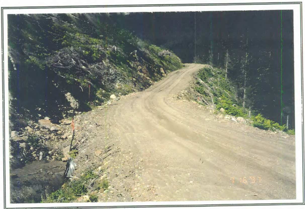
PHOTO H5. Sand road adjacent to the mainstem channel with full sump above cross drain [Site H7].
