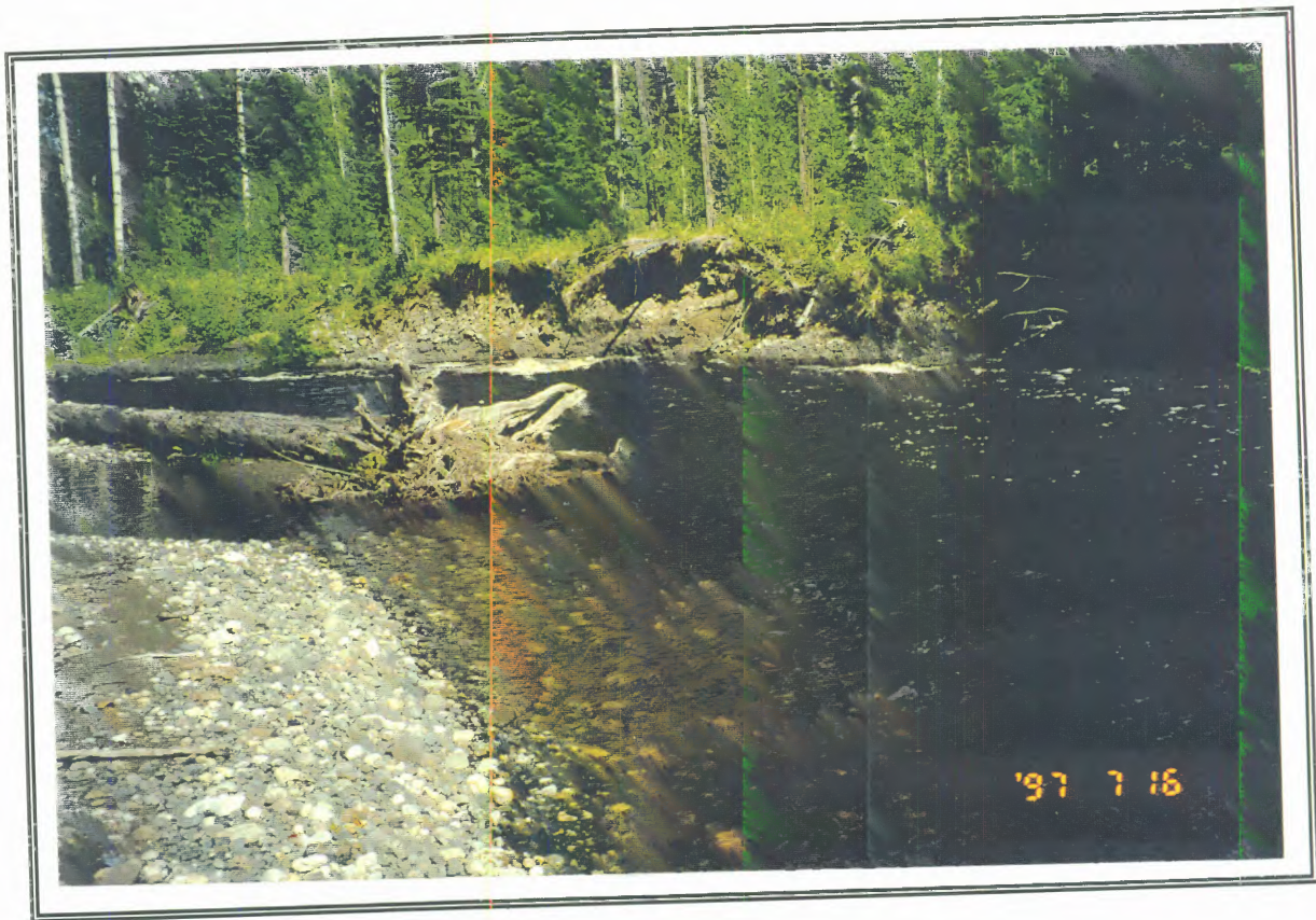
SITE M2. Moffat Creek, approximately 2 km upstream of site M1. Note the bank erosion.
