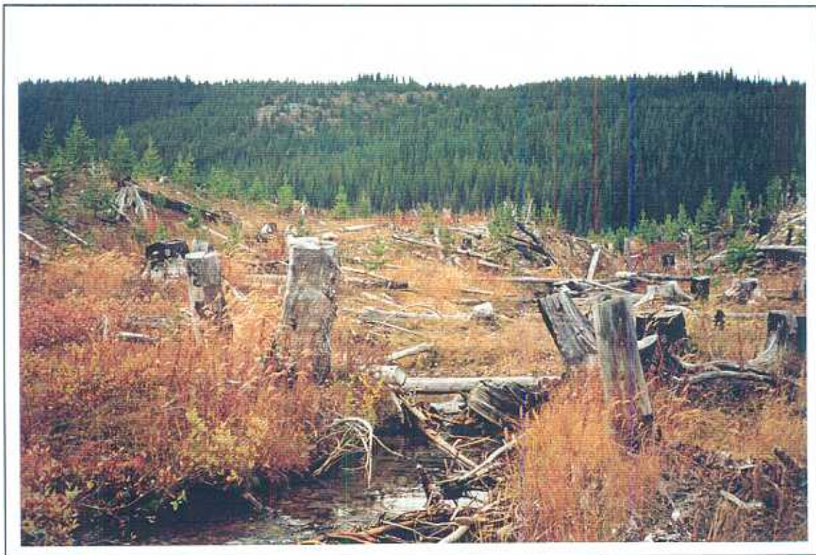
Photo 72: Granite Creek. View of Site 4 upstream of culvert facing upstream. Note clearcut and undercut banks (6 October 1996).
