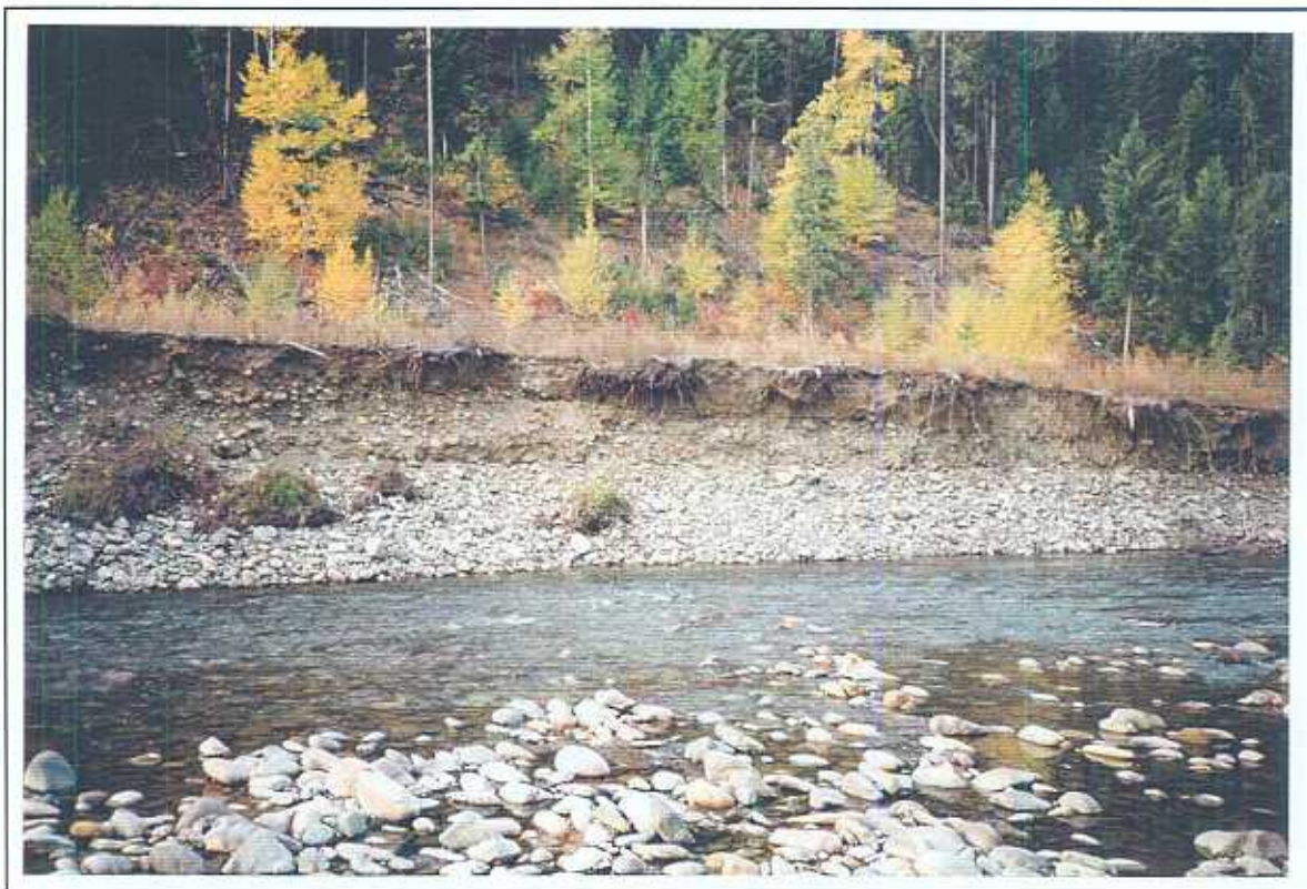
Photo 6: Tulameen River. View of Site 2 facing right bank. Note eroding banks. (4 October 1996).
