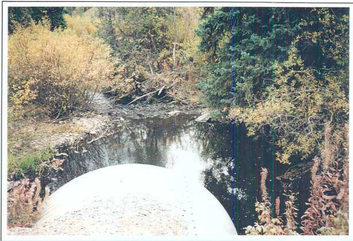
Photo 113: Otter Creek. View of Site 5 facing upstream. Note pool upstream of culvert. (3 October 1996).
