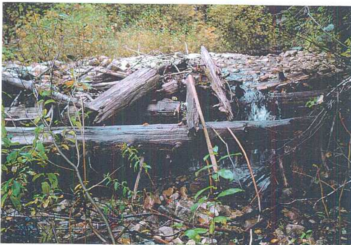
Figure 4.5. Collapsed crossing and sediment wedge, reach 11.
