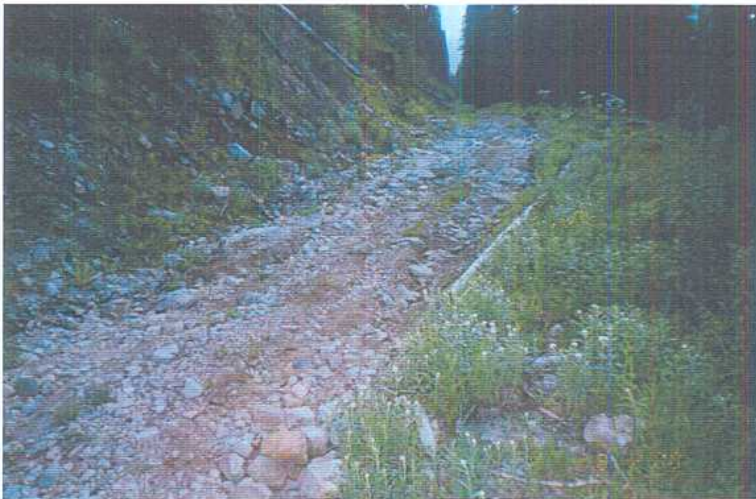
Plate 14: Rutted road surface at 12.1 km along Sitkum Creek FSR.
