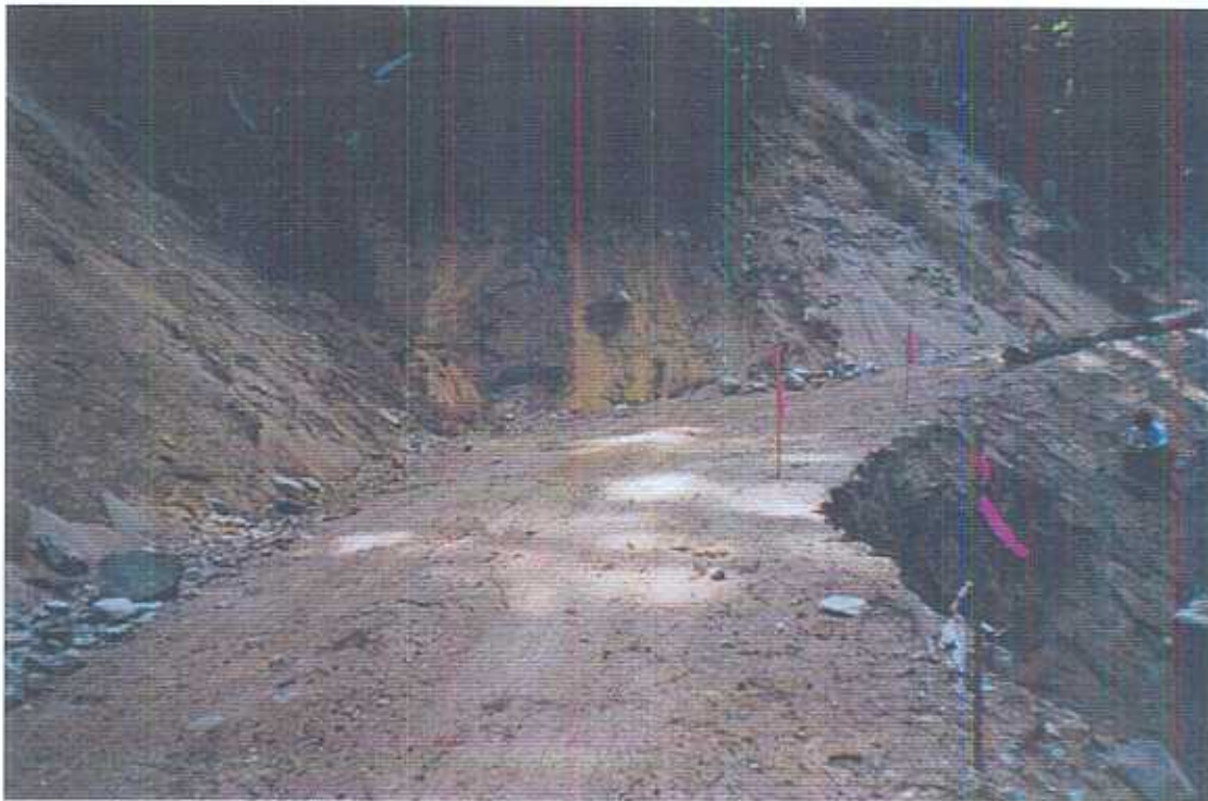
Plate 11: Road fillslope failure (S13) at gully crossing of Sitkum Creek FSR at 8.75 km. Note 2-3 m vertical headscarp at right. Date: 02-Aug-2000 Photograph 4-15
