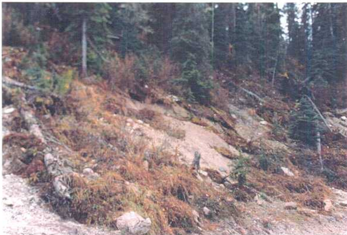
Figure 4 Mass wasting site on upper side of road at approximately 61 km on Raft Road 9.
