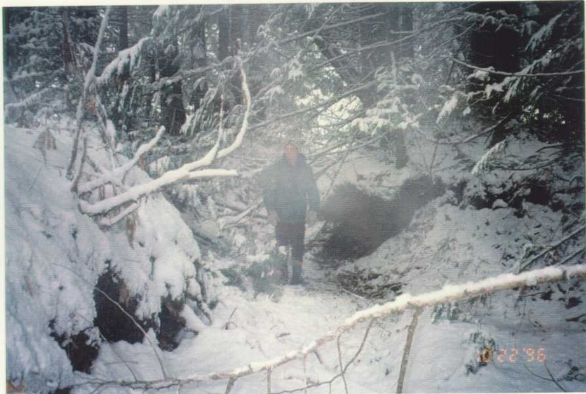
Eroding banks downstream of culvert in Reach 1, tributary 9 to Monashee Pass Creek. The banks downstream of the Monashee Pass FSR culvert are composed of road gravel fill eroded from upstream. The culvert is damaged and partially filled with gravel.
