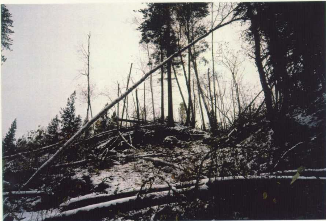
Slumping banks adjacent to Reach 2, Yeoward Creek are related to a trail parallel to the north side of the creek, a landing and old upslope logging. Bank stabilization with rooting vegetation is recommended, however soils are fine colluvium and trees have been easily uprooted.
