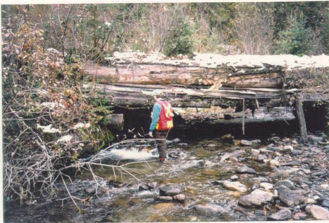
The bridge has vegetation growing on it, rotten stringers, 3 of 4 abutments are eroded, the bridge is sinking and sediment is evident in the channel. The bridge requires removal.
