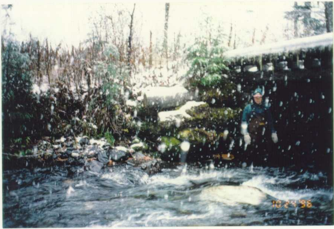
View of bridge crossing and abutment in Reach 6B, Monashee Creek which is a human impact to the channel.
