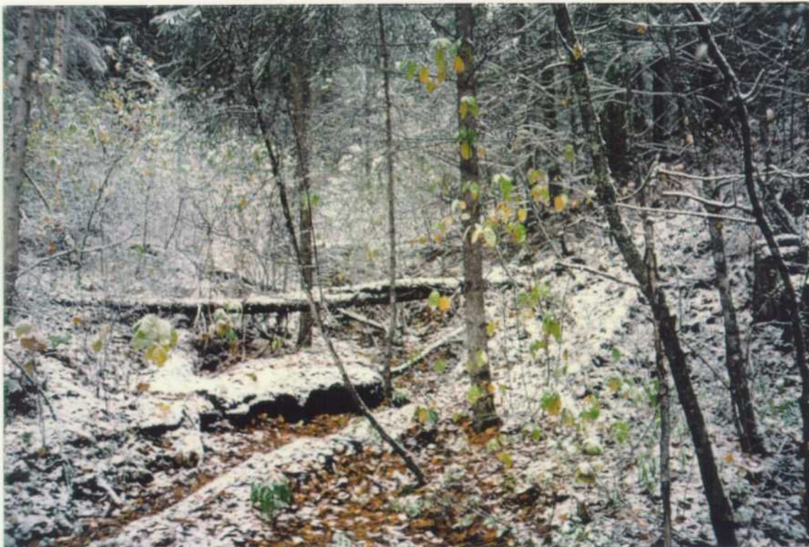
Cedar Gulch is dry in reach 2 upstream of Hwy. 6. There is sign of high flows indicated by the sediment deposit at the upstream end of the highway culvert.
