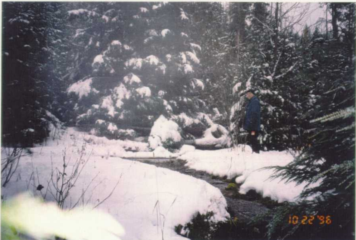
On the access road to site 2660 an old wooden culvert is not functioning and the creek is flowing over the road. The culvert should be unplugged or replaced.
