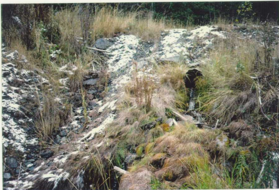
Culvert draining Reach 1, Half Mile Creek under Hwy. 6. The creek forms multiple channels immediately downstream of the culvert under the powerlines. The creek becomes a single channel when it re-enters the young, coniferous forest. Upstream of Hwy. 6 the channel is functioning well in a mature coniferous forest.
