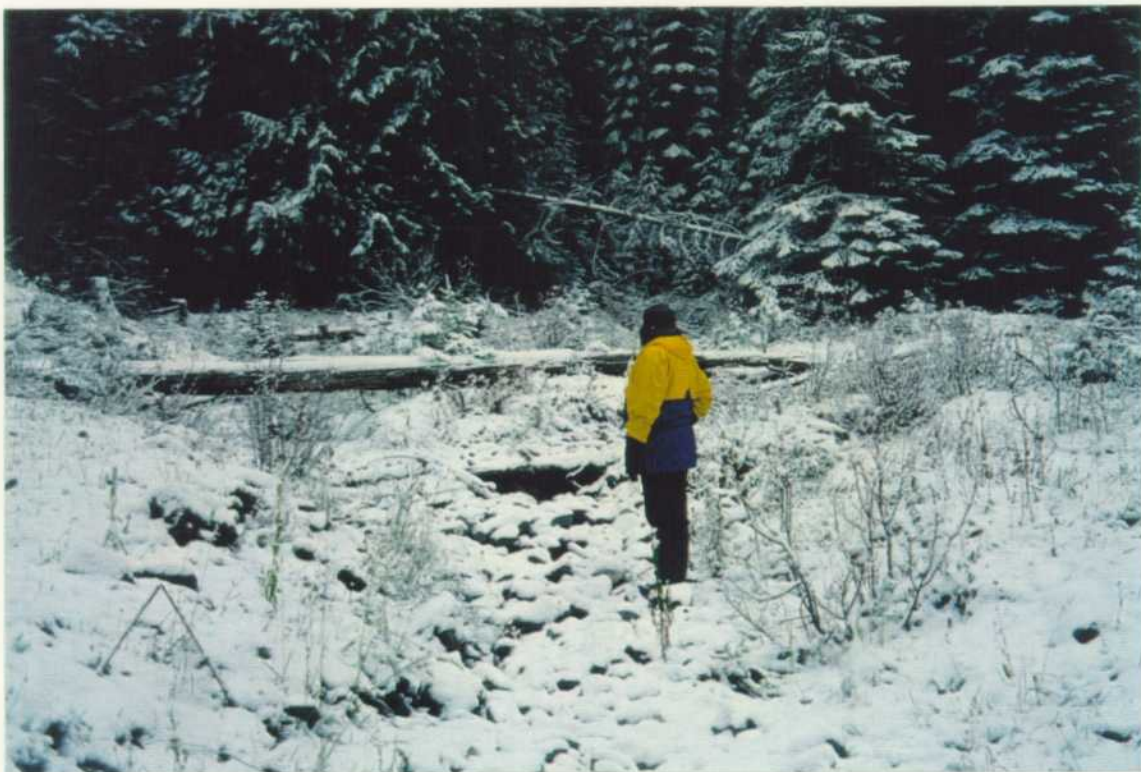
Upstream view of Reach 1, Tributary 6 to Monashee Pass Creek shows the disturbed stonelines. In addition, downstream of the photo there is a culvert which is out of alignment with the stream channel and is causing erosion and a sediment source.
