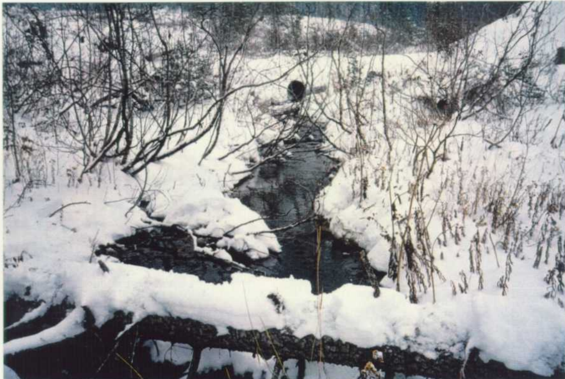
Upstream view of culvert and Reach 3, Yeoward Creek. Abundant silt in the creek indicates aggradation.
