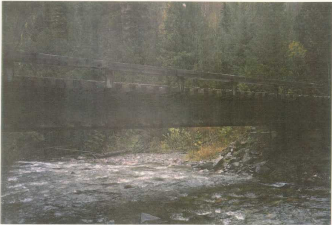
The bridge crossing to the Yeoward sub-basin is sound, however, aggradation of the channel is occurring in the vicinity.
