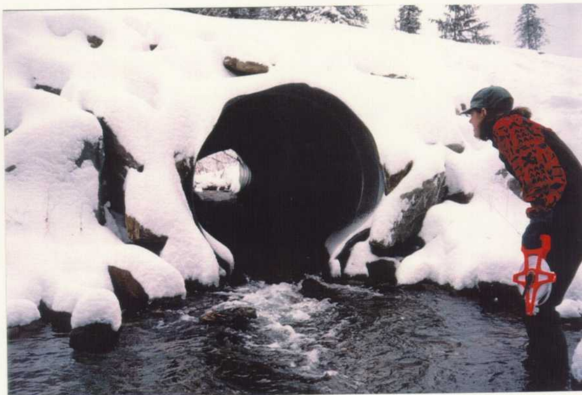
View of the dented culvert at the Yeoward road crossing. A possibility for culvert failure exists.
