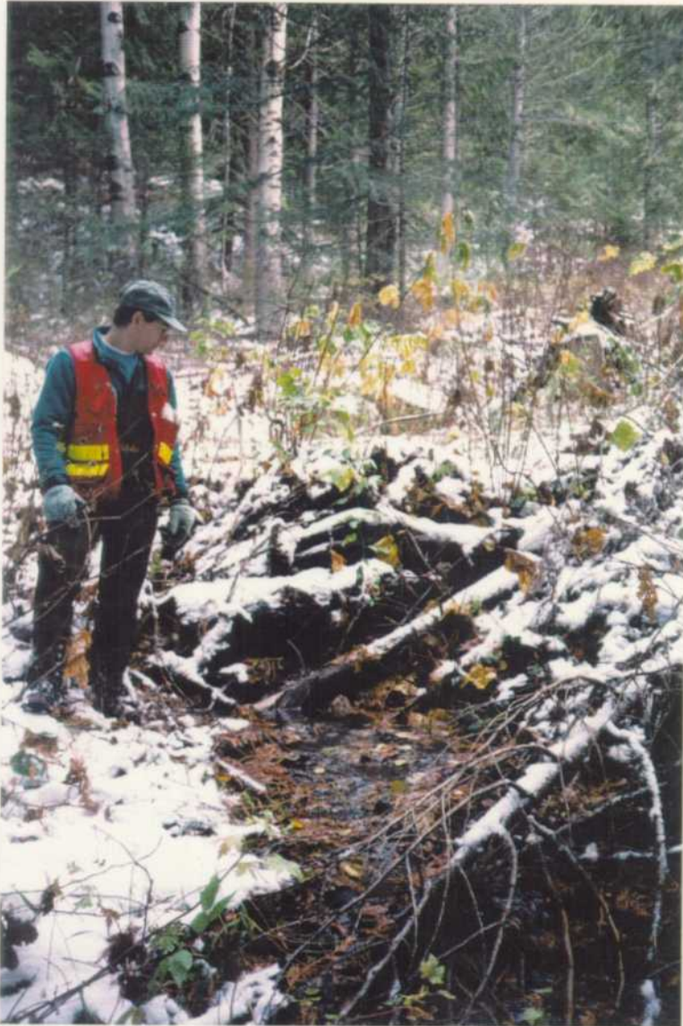
View of collapsed bridge. In order to reduce the aggradation process the bridge should be removed. In addition, the adjacent landing should be revegetated to stabilize the soils.
