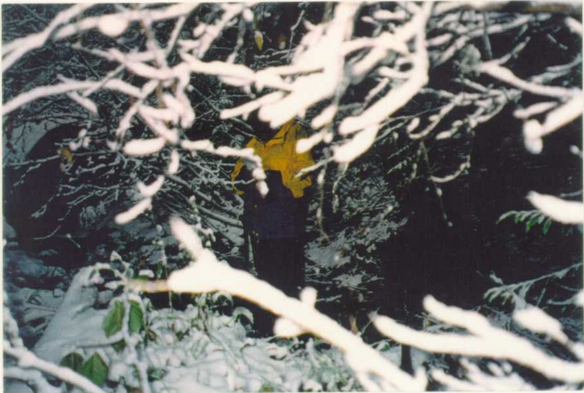
The banks are eroding at the downstream end of the culvert as a result of its misalignment.
