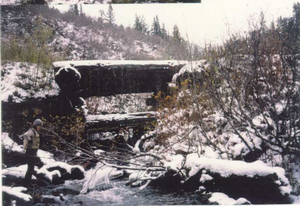
The bridge crossing consists of two bridges on top of one another. The channel is narrowed by the abutments and if any failure occurs there will be a large impact to the creek, therefore, the bridges should be removed.
