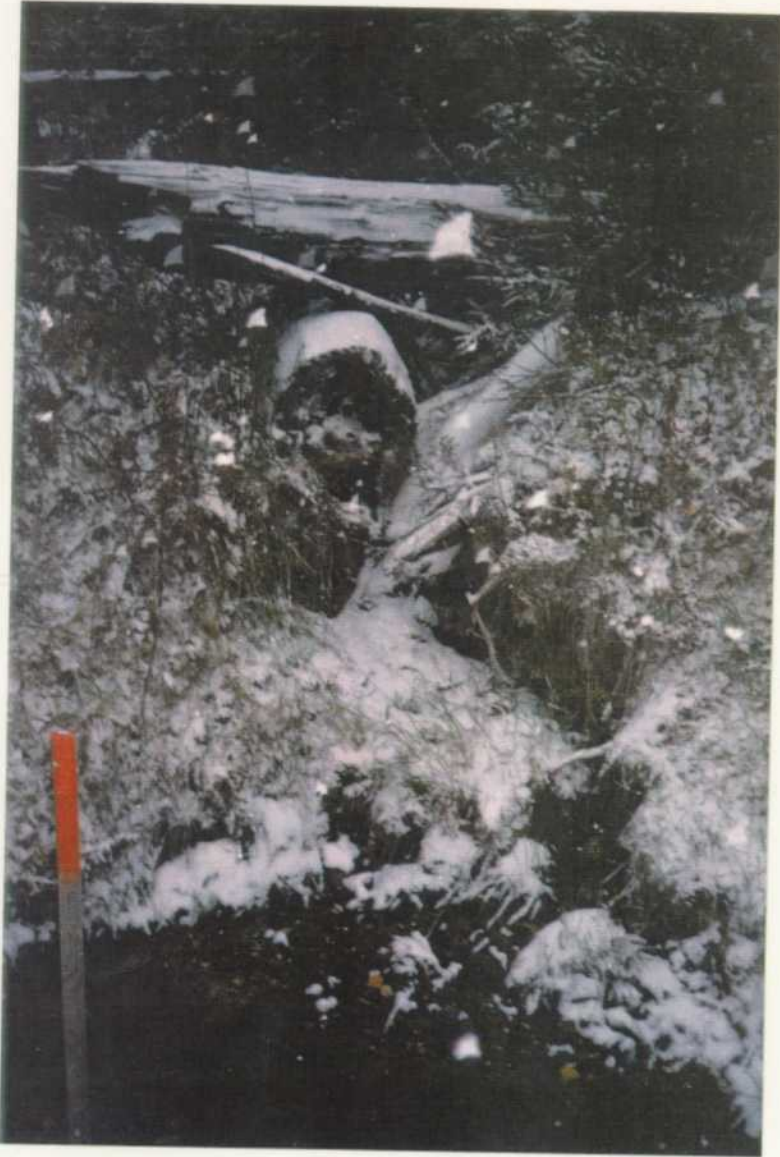
Upstream view of Reach1 of Tributary 9 to Railroad Creek shows the sediment in the settling pool. Sediment is predominant throughout the channel system.
