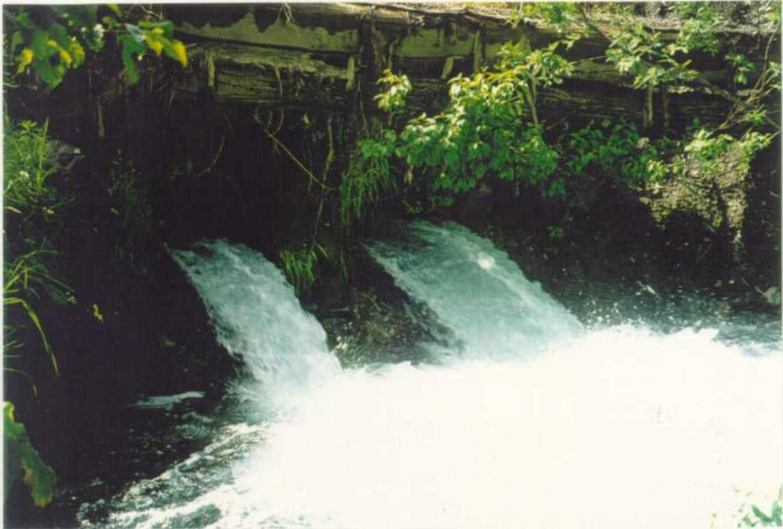
Reach 2, Site 2 of Monashee Pass Creek, fish passage barrier is a 0.8m culvert under Hwy. 6.
