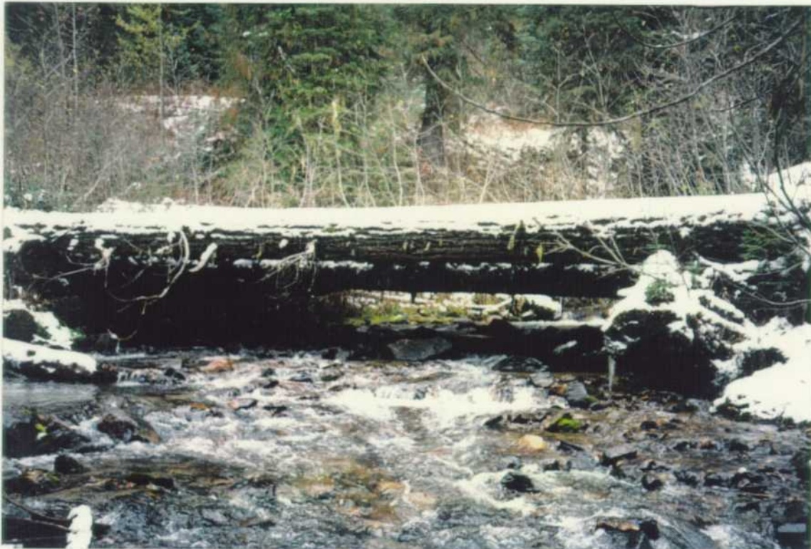
Upstream view of Reach 8B, Monashee Creek shows an abandoned bridge with a rotten deck.
