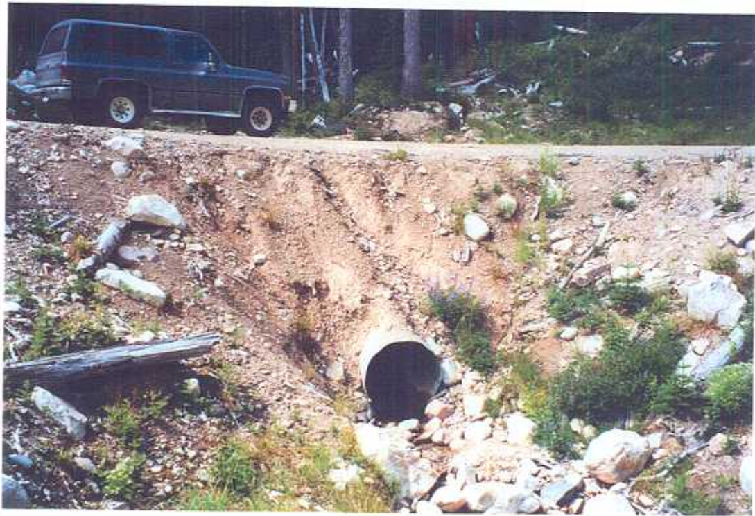
Photo 22: Raveling at fillslope to culvert outlet, SS10.
