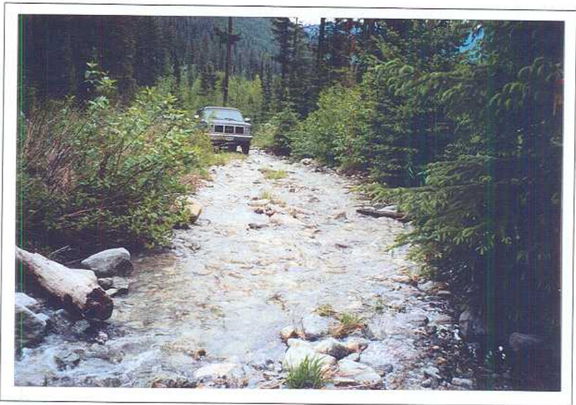
Photo 18: SS1. Flow diverted over road.
