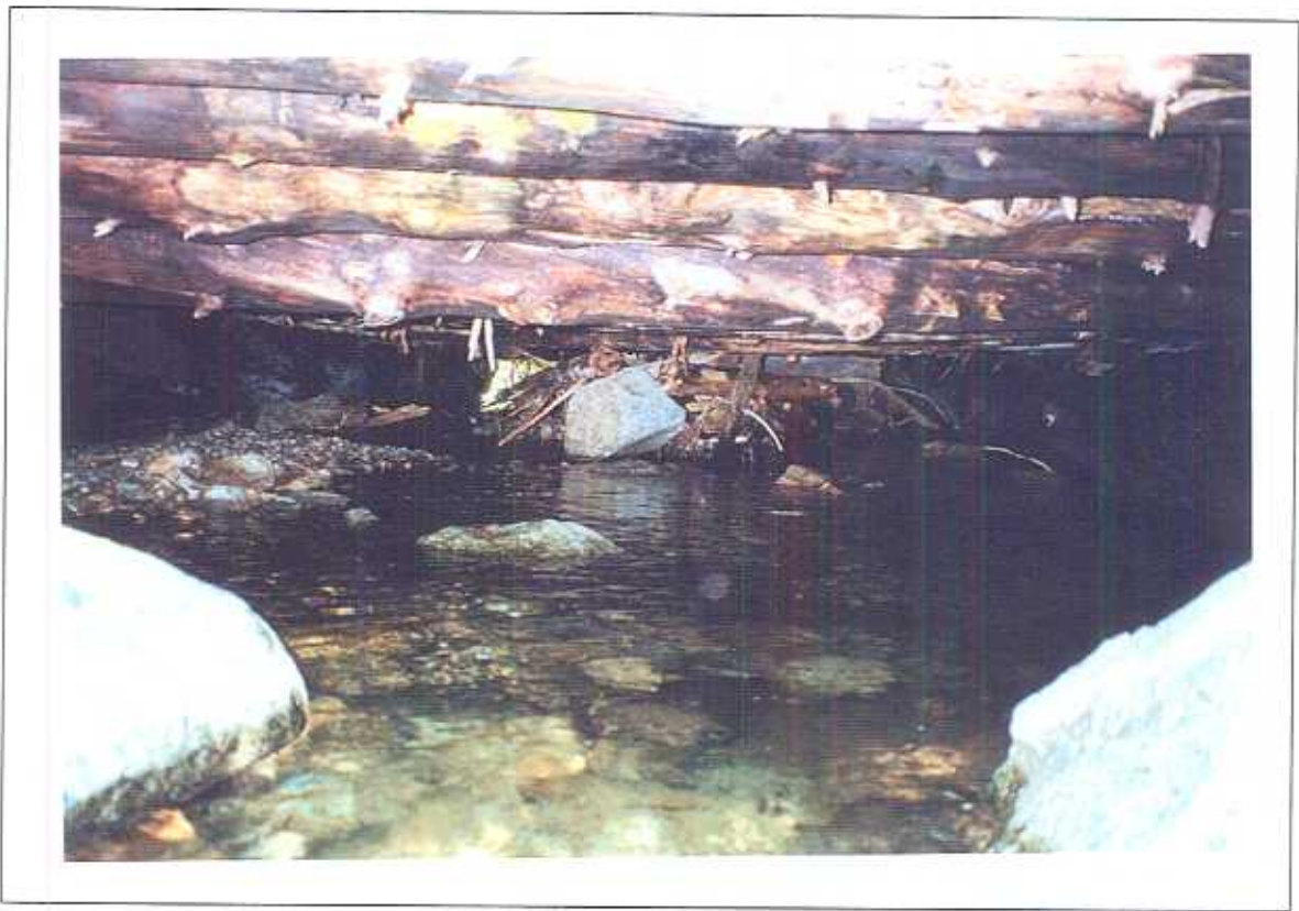
Photo 20: Collapsed structure in July Creek.
