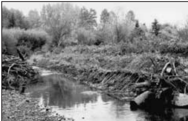
Figure 6. Brush mattress and willow wattles stabilize a streambank that was recontoured to reduce active erosion.
